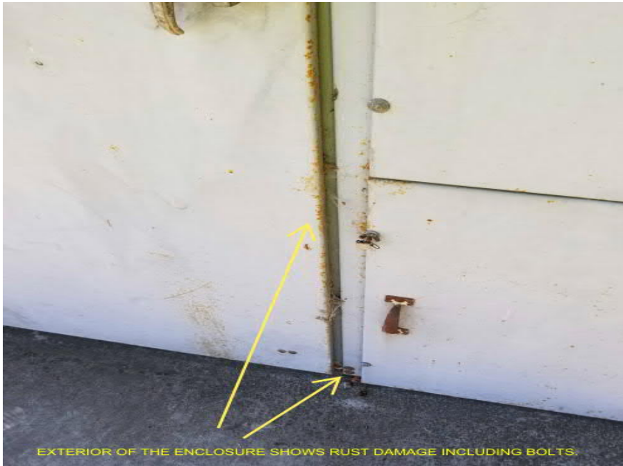
Photo E- 4 Exterior Service Entrance Switchboard Skin Door.
