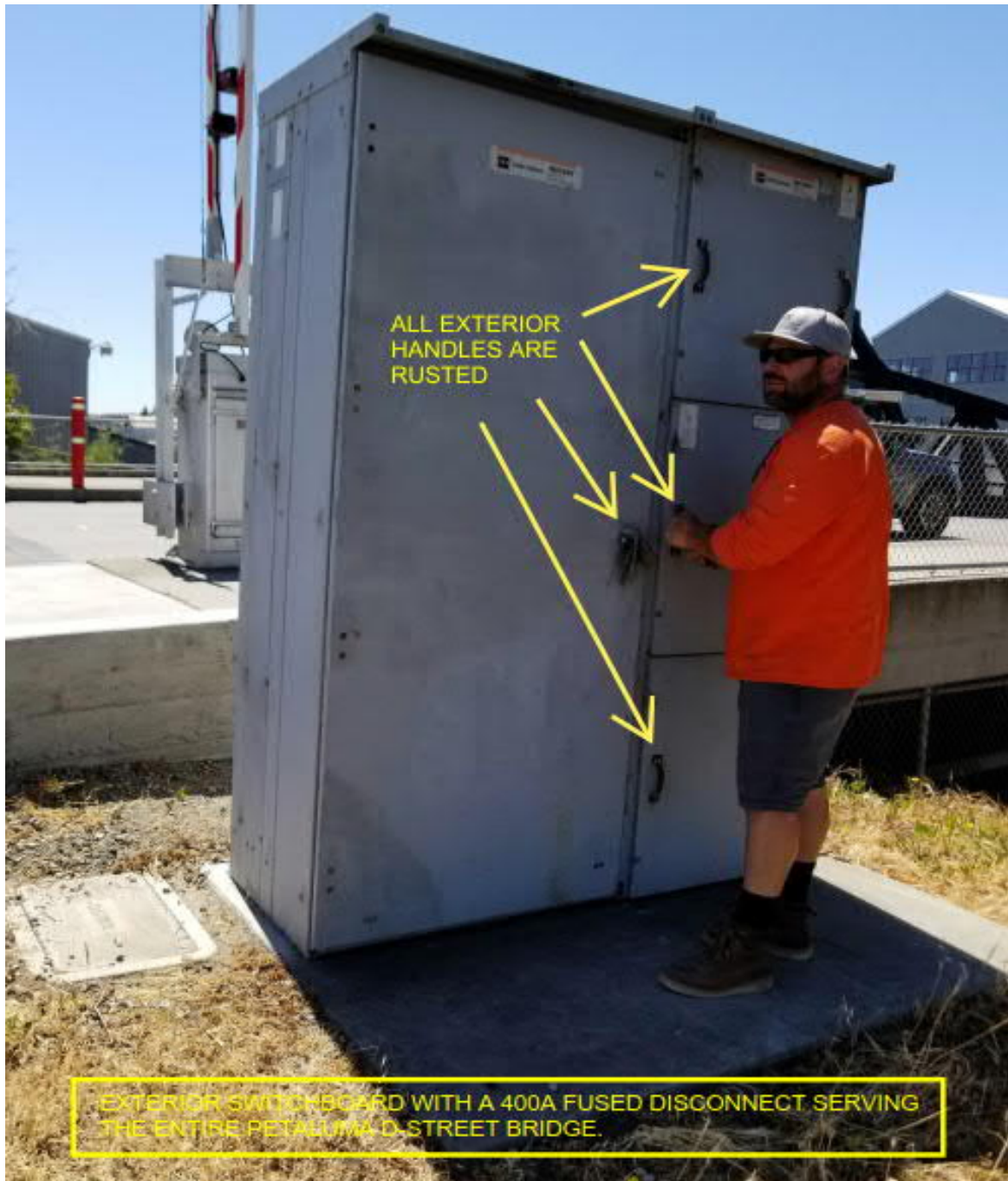
Photo E- 1 Exterior Service Entrance Switchboard
