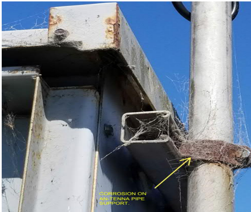
Photo E-6 Wireless Antenna Pole Support Fastener at MCC-2.
