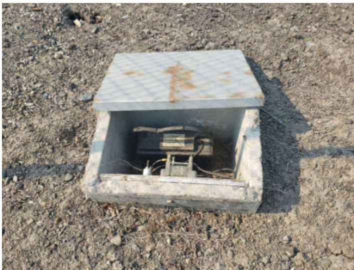
Photo #18: Concrete vault with battery and electrical connection
