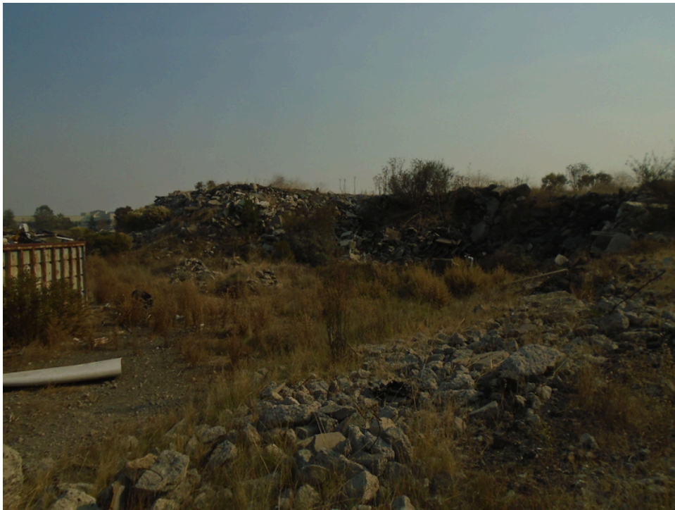
12. View of the construction debris piles
