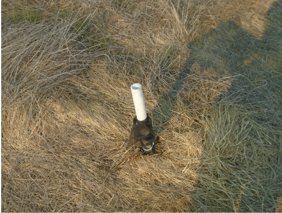
7. View of a possible monitoring well observed on the northeast portion of the property
