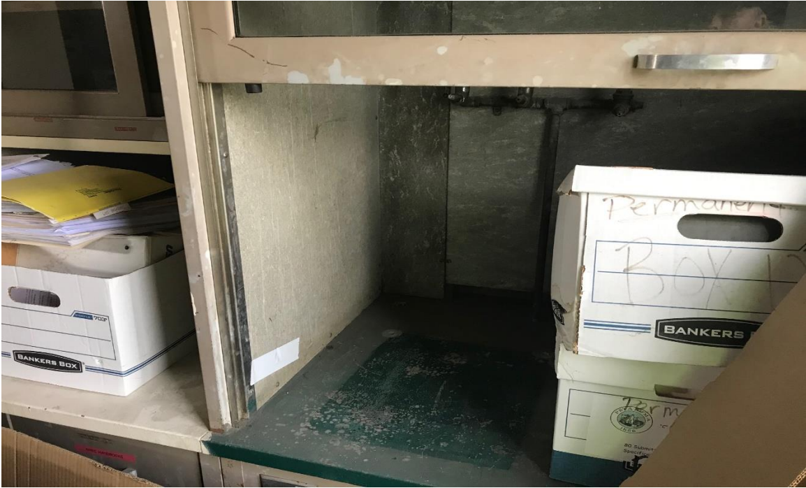
Asbestos cementitious “transite” hood panels in the lab of the Operations Building
