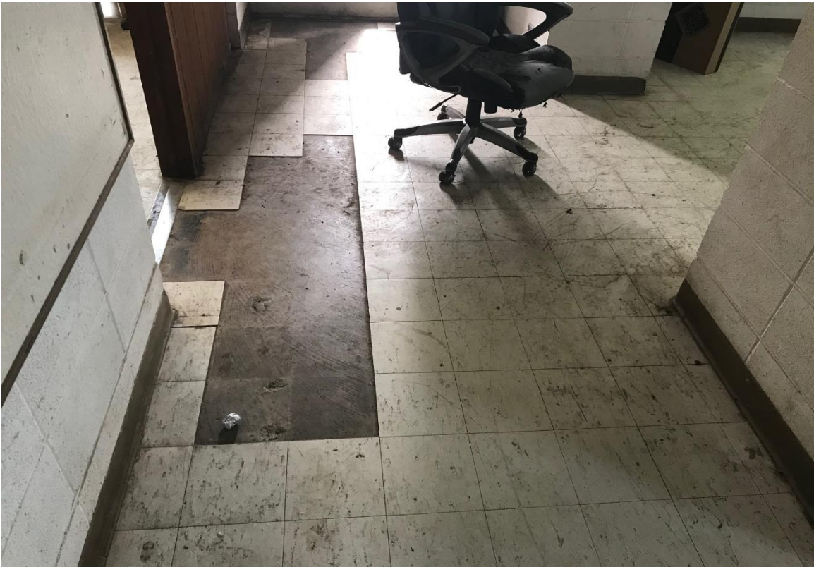
Asbestos containing 9” vinyl floor tile w/black mastic in the Operations Building
