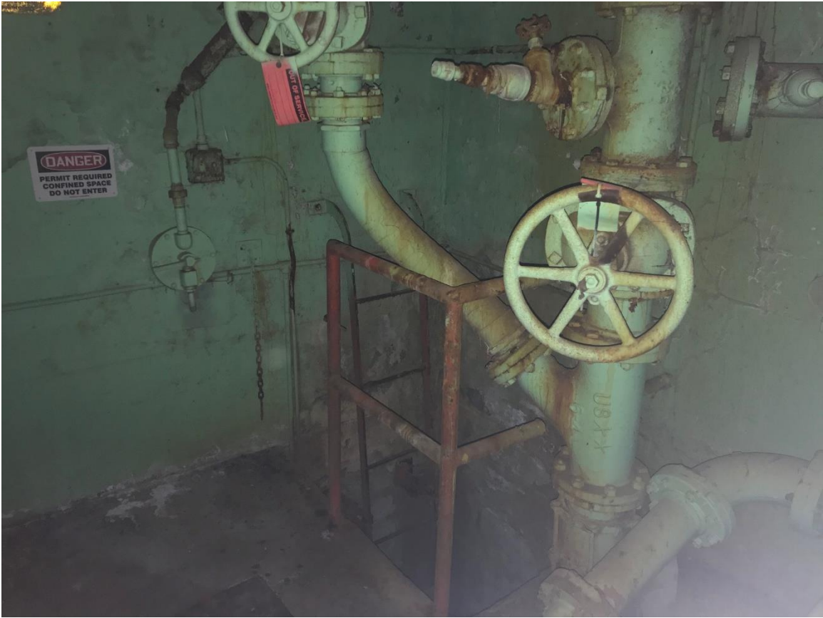
Lead based interior green concrete wall, green metal ladder to pit, and red metal railing on the lower level of the Secondary Digester
