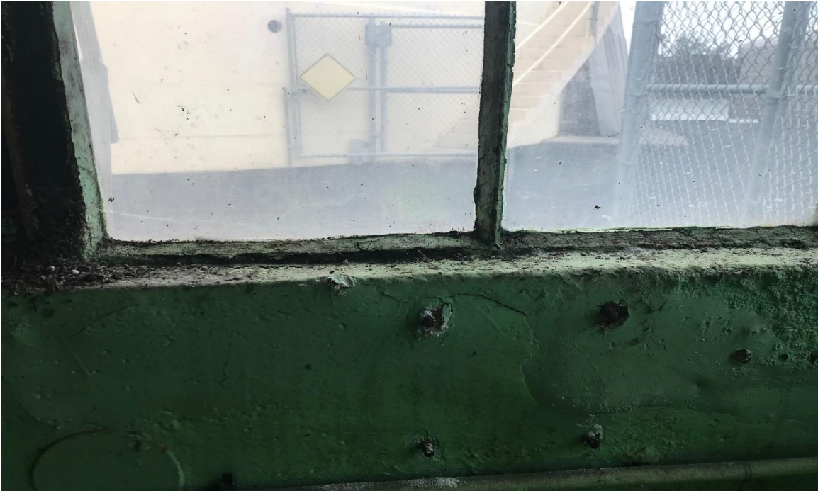
Lead based interior green metal windows of the Secondary Digester
