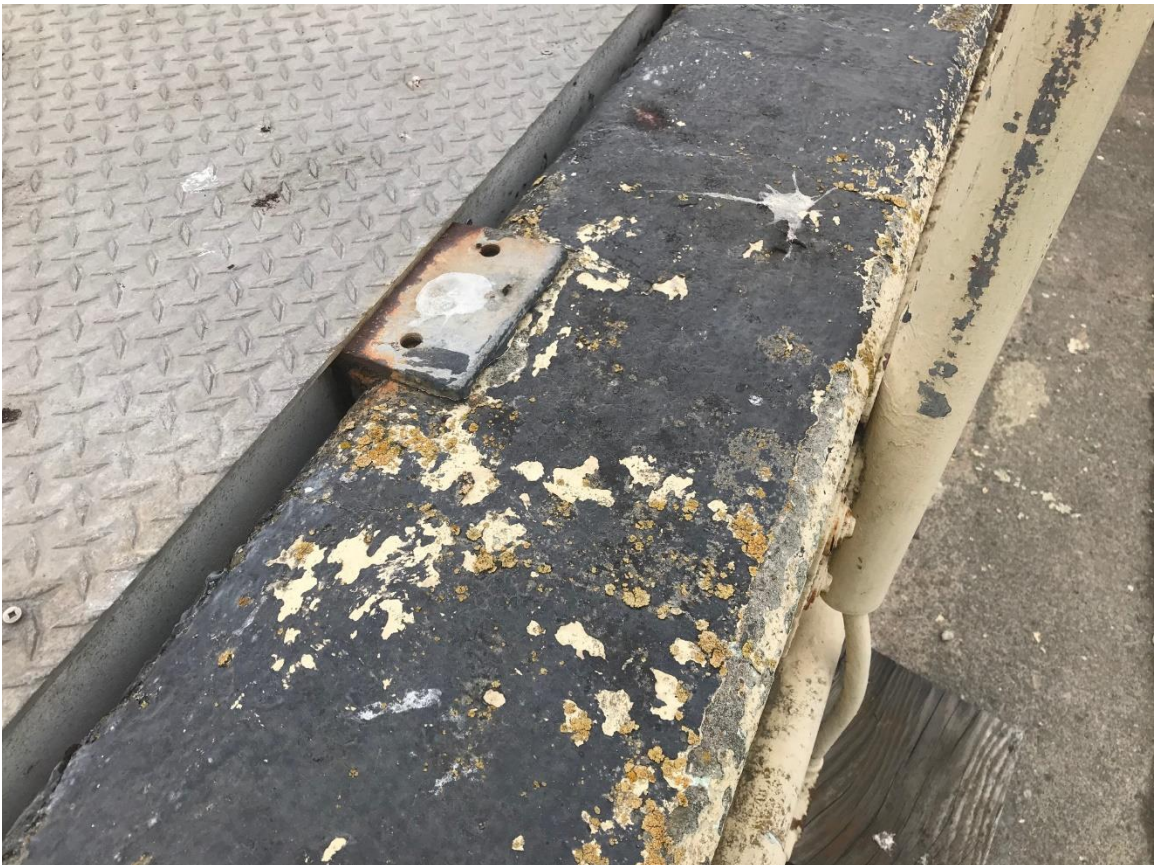
Asbestos containing black mastic on the raised portion on the roof of the Secondary Digester
