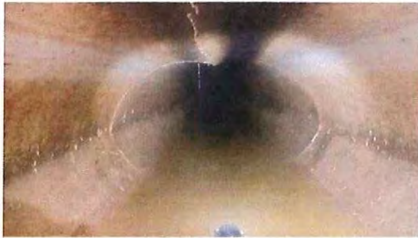
220' pipe is collapsing. Hinge cracks visible at 12, 3 and 9 o'clock
