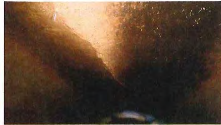
From 210'-225' compression damage at top of pipe. Pipe is collapsing.
