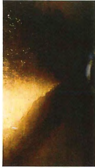
From 210'-225' compression damage at top of pipe. Pipe is collapsing.
