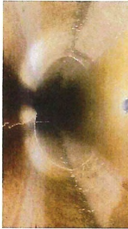
220' pipe is collapsing. Hinge cracks visible at 12, 3 and 9 o'clock
