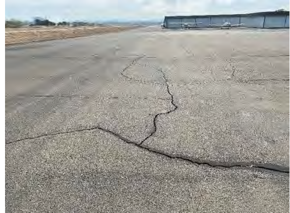
Photo 2: Block Cracking in North Section
