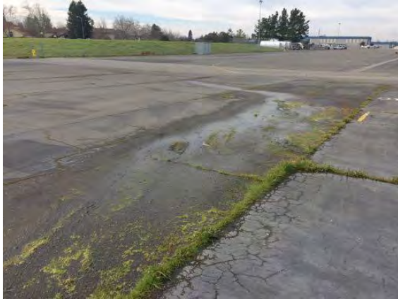
Photo 1: Depression and Ponding in South Section
