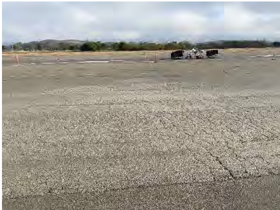
Photo 5: Alligator Cracking in South Section
