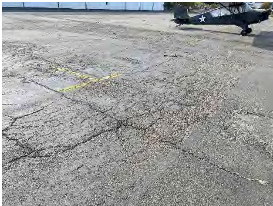
Photo 3: Raveling of Pavement
