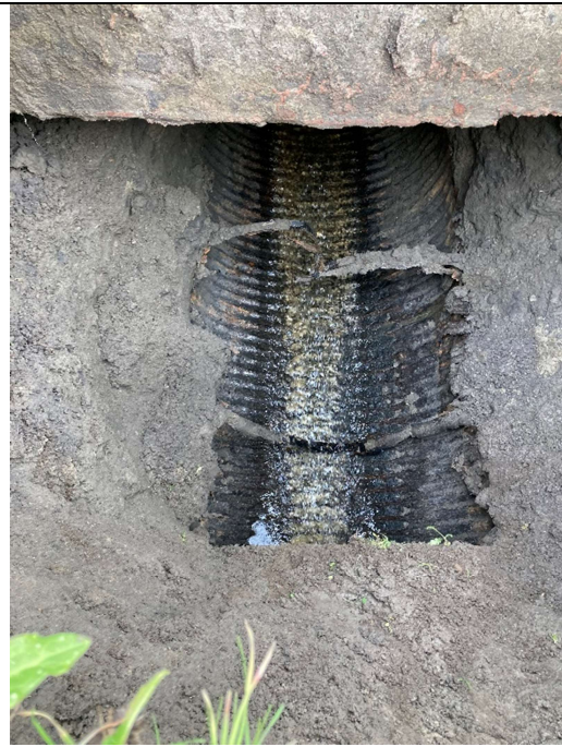
Exposed sinkhole location 48" CMP
