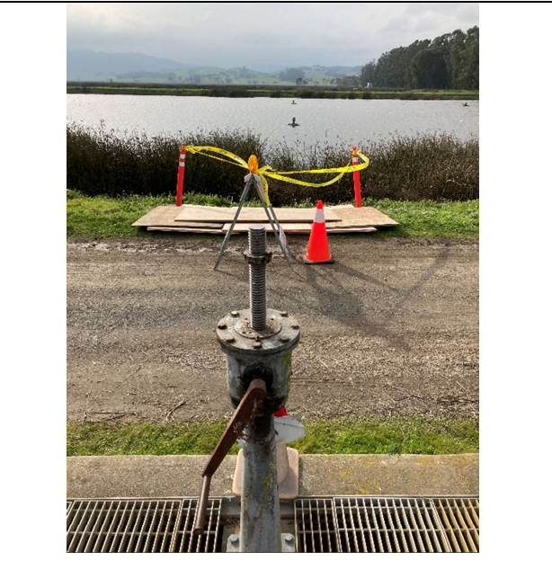
Standing on top of transfer structure looking towards sinkhole and Pond No. 4.
