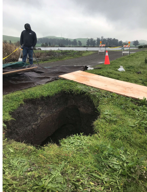
Sinkhole and Pond No. 1 in background.
