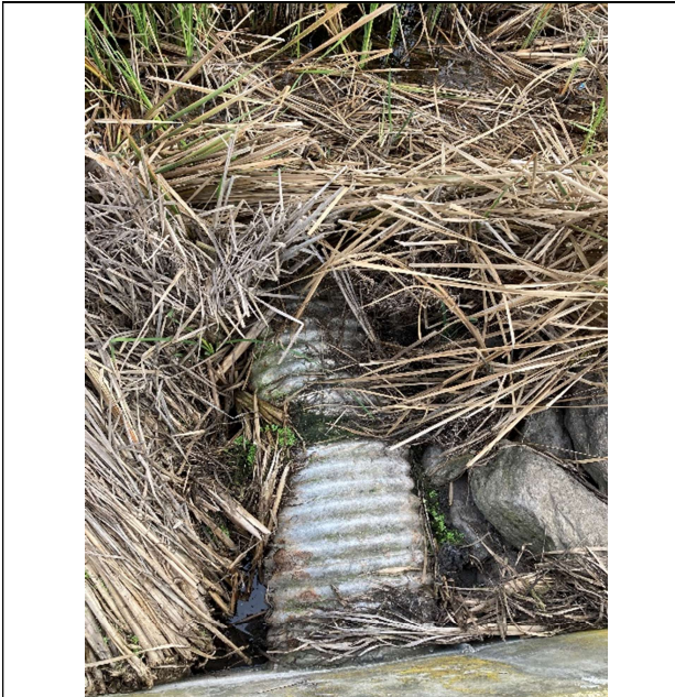
24" CMP Inlet that transfers flow on Aerated Lagoon side.
