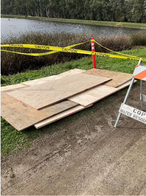
Sinkhole and Pond No. 4 in background.
