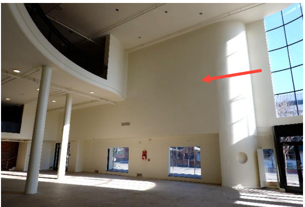
Figure 11. Narrow enclosed storage rooms are located at the mezzanine and second story along the east and south walls (indicated by red arrow).
