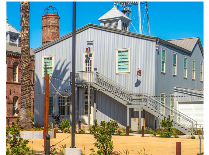
EXISTING METAL STAIR NEW LANDING TO MATCH COLOR & DESIGN OF EXISTING - SUBMIT SHOP DRAWINGS TO VERIFY
