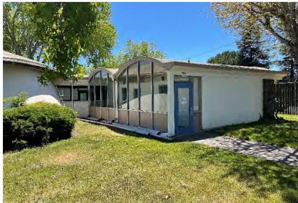
Figure 41. Restroom and kitchen addition (Phase II of original construction) with a barrel-vaulted roof at the west side of the Herzog Hall.
