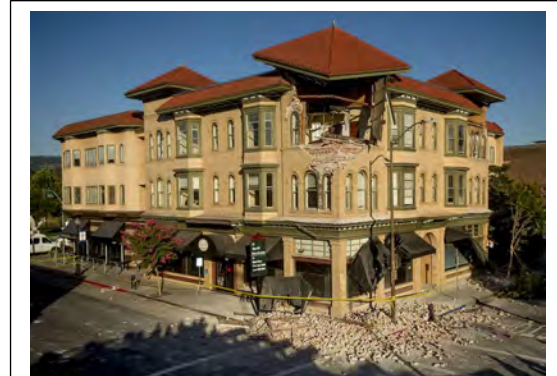
In 2014 a 6.0 magnitude earthquake occurred in the southern portion of the City of Napa on the West Napa Fault. The event was the largest earthquake in the San Francisco Bay Area since the 1989 Loma Prieta earthquake. Total damage in the southern Napa and Vallejo areas ranged from $362 million to $1 billion. Photo Credit: LA Times 2014
