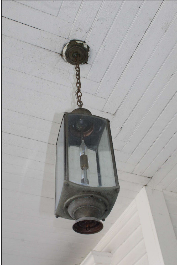
Photo 12 – Light fixture, porch
