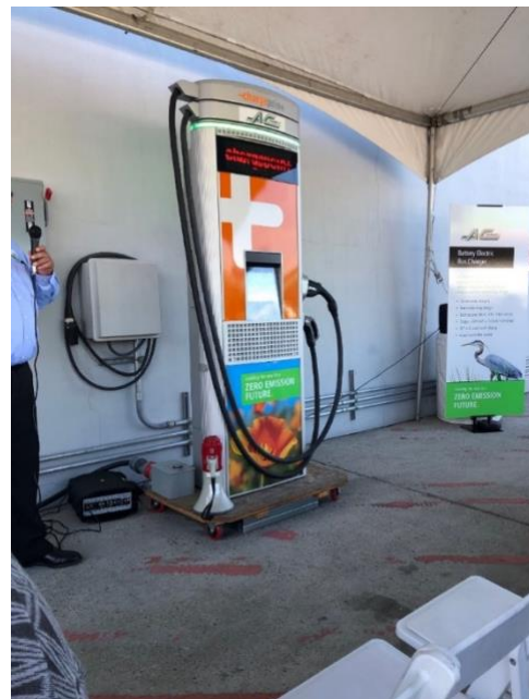
An electric bus charger in use by AC Transit, Division 4
