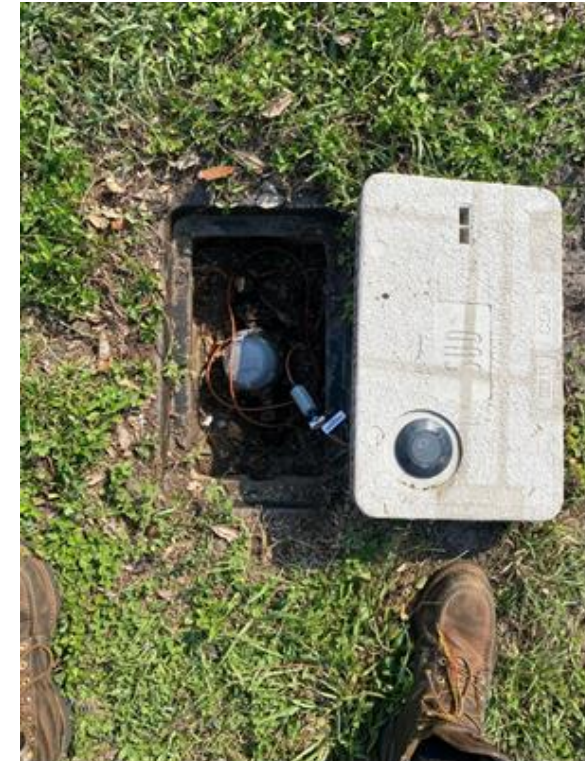
Water meter inside water meter box
