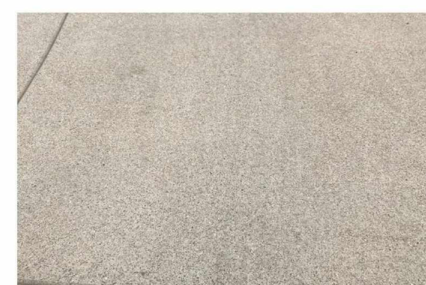
P1 C.I.P. CONCRETE PAVEMENT MATERIAL: CAST-IN-PLACE CONCRETE COLOR: STANDARD GREY FINISH: TOPCAST #05 "SANDBLAST" JOINT: SAWCUT
