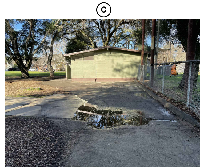
(E) TRANSITION FROM AC TO QUARRY FINES PROTECT QUARRY FINES PATH IN PLACE
