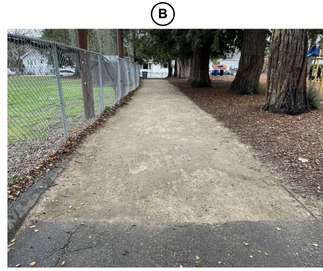
(E) TRANSITION FROM AC TO QUARRY FINES PROTECT QUARRY FINES PATH IN PLACE
