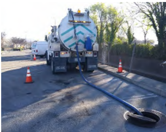
Figure 12: Drain hose decanting water from Combination sewer cleaning truck
