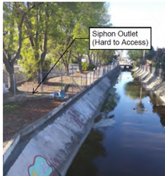
Figure 3: Poor access to outlet structure
