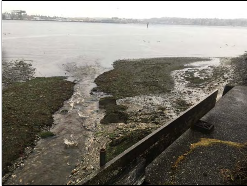
Photograph 1. View north from the Bay Street Bridge. Annapolis Creek empties into Sinclair Inlet.
