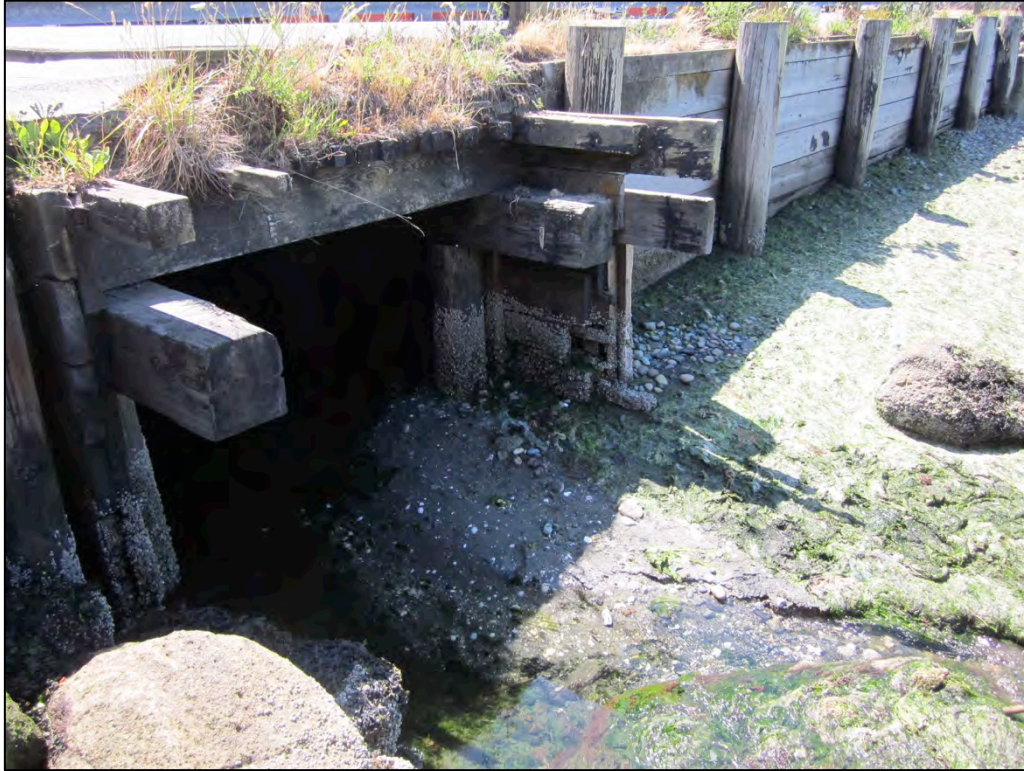
Figure 3. Timber trestle and bulkhead located at Bay Street at the outlet of Annapolis Creek; view is to the southwest. If these are historic in age they would need to be recorded and evaluated prior to replacement.
