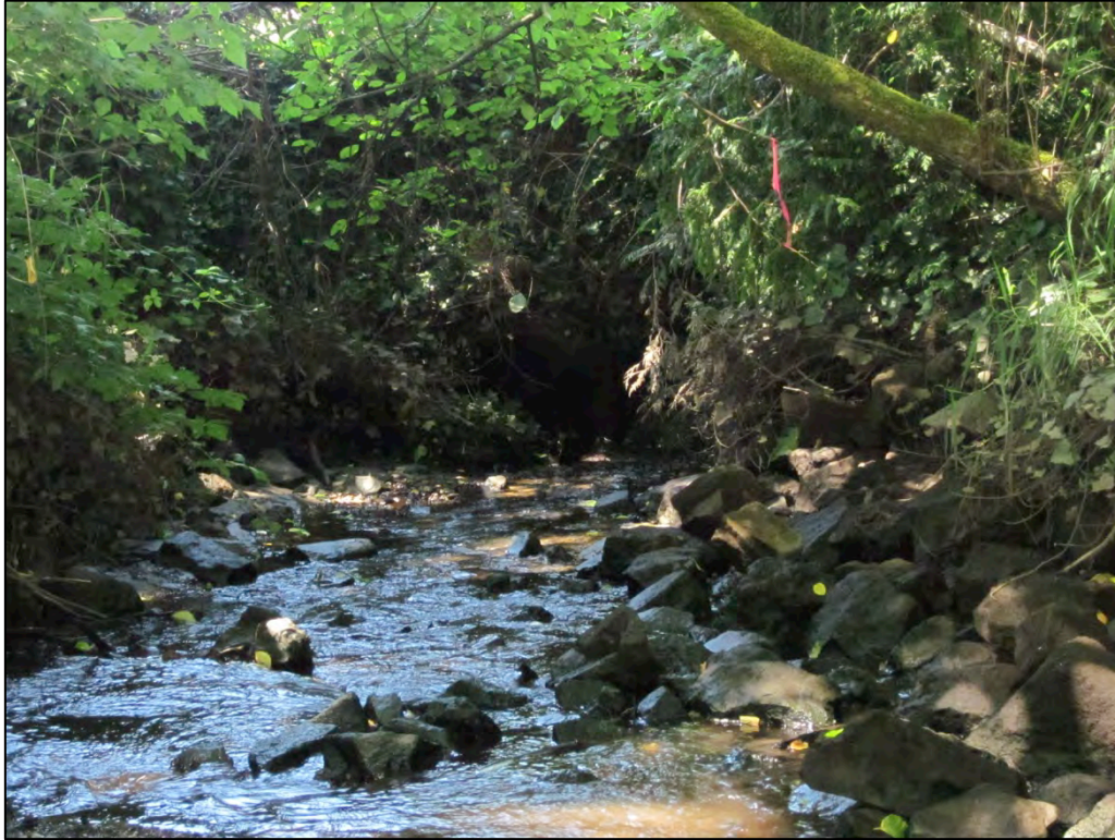
Figure 5. Culvert carrying Annapolis Creek under Bay Street; view is to the north-northwest. Bank is armored in foreground.
