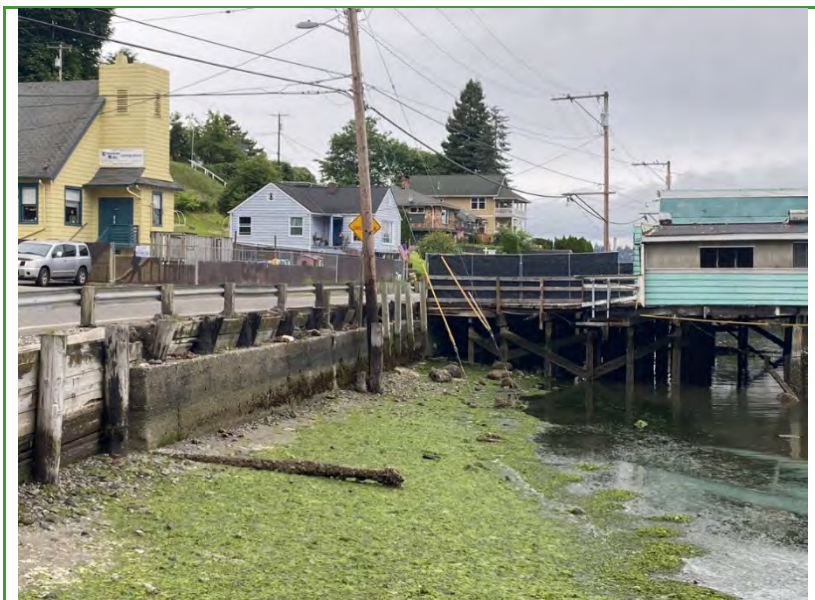
Failing armor on Bay Street near Annapolis Creek.
