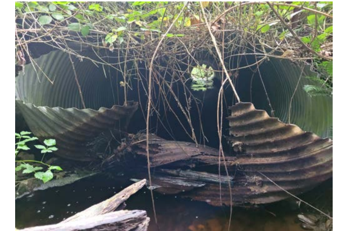
Damaged culvert inlet
