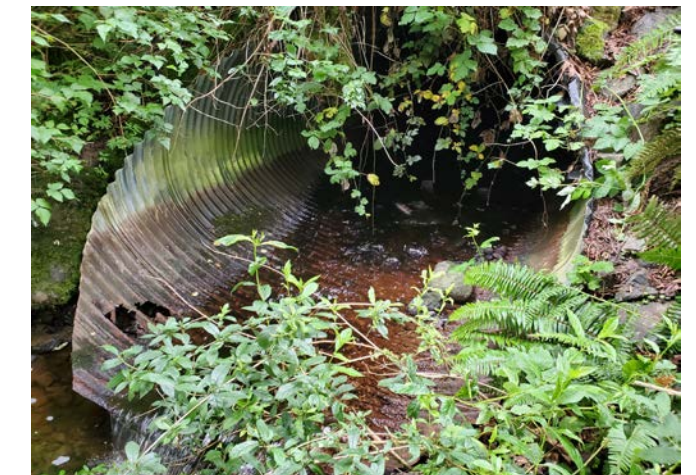
Rusted culvert outfall with short water surface drop
