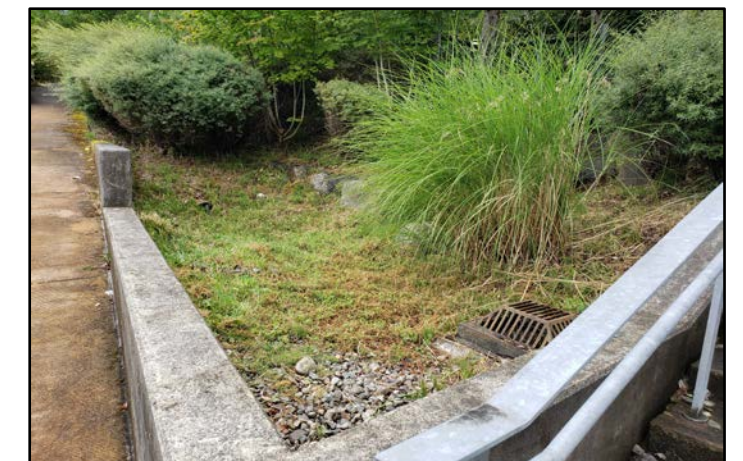
One of two water quality facilities in Downtown Basin
