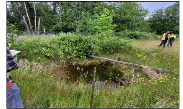
Sinkhole on property from damaged culvert
