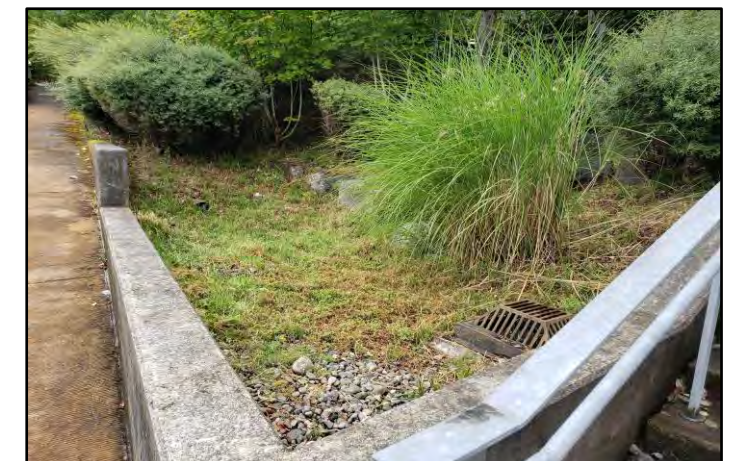
One of two water quality facilities in Downtown Basin
