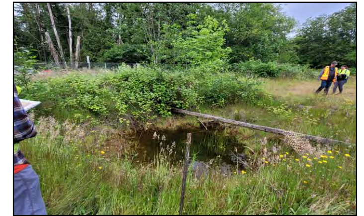
Sinkhole on property from damaged culvert
