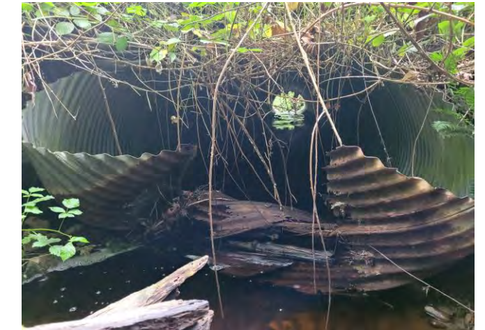
Damaged culvert inlet
