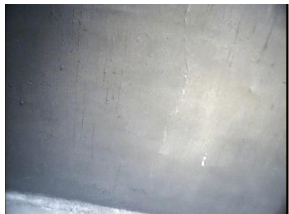
(#23) Wall Crack Quadrant 4
