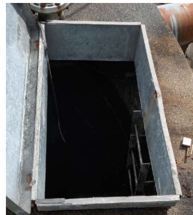
(#12) Roof Access Hatch Gasket
