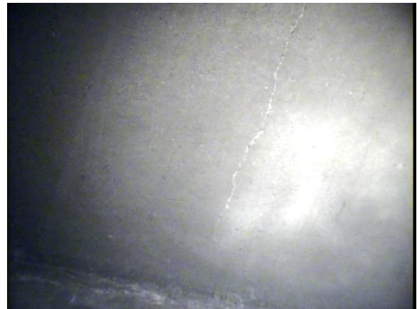
(#22) Wall Crack Quadrant 3
