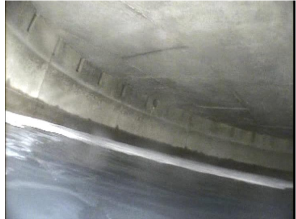
(#10) Ceiling 3 O'clock / Overflow
