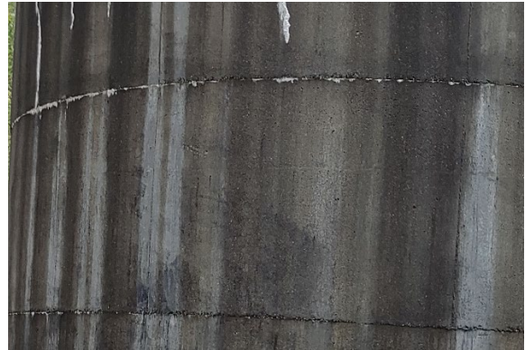
(#4) Exterior Shell Seam
