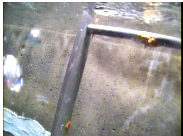
(#18) Interior Ladder Rust Nodules
