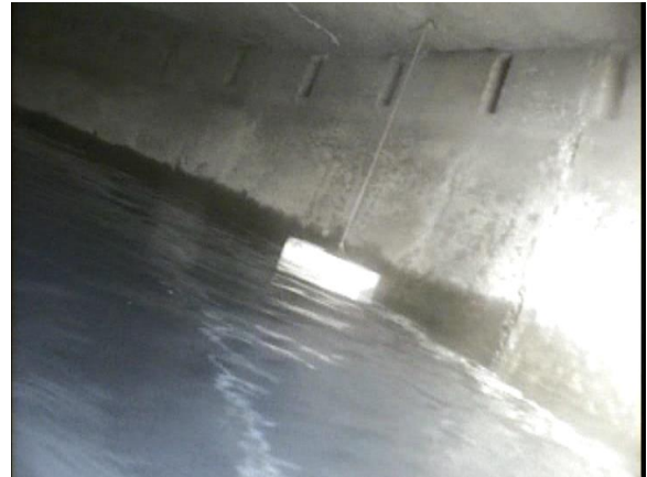
(#16) Ceiling 9 O'clock / Float
