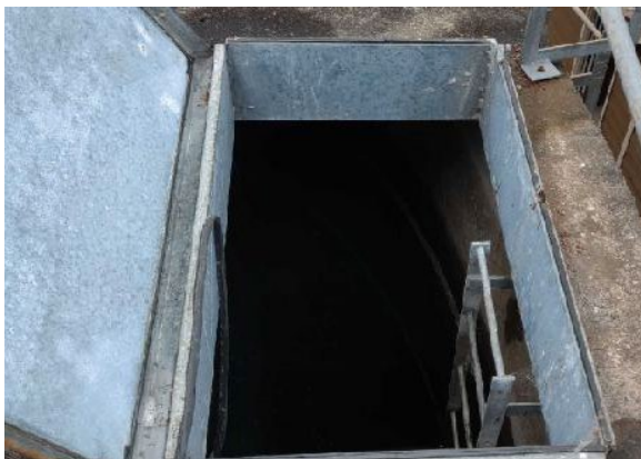
(#9) Roof Access Hatch Gasket
