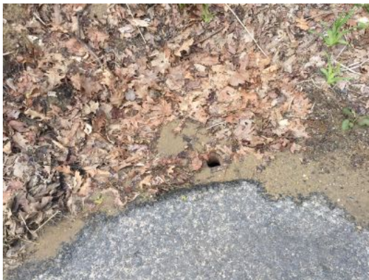
Storm Drain Clogged with Sand, photo courtesy of CBH
