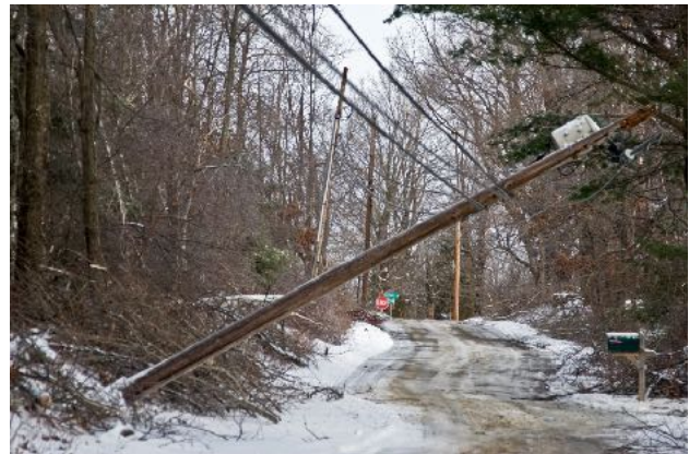
Storm damage, photo courtesy of CS
