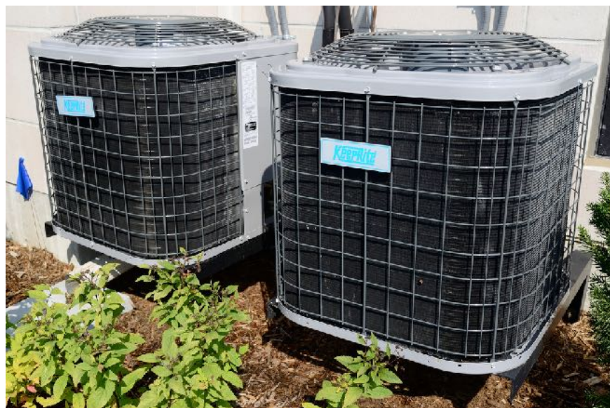
Air Conditioning Units, photo courtesy of Pixabay
