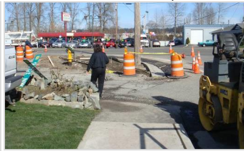
Does Not Meet ADA Requirements
