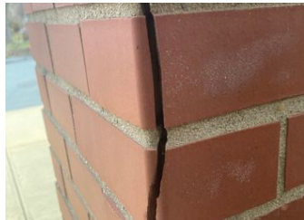
Brick Facade cracks
