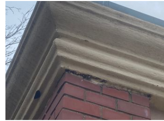
Stucco Eifs - Cornices decay
