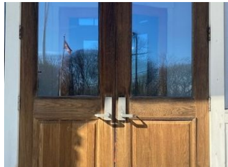
Side Entrance Doors
