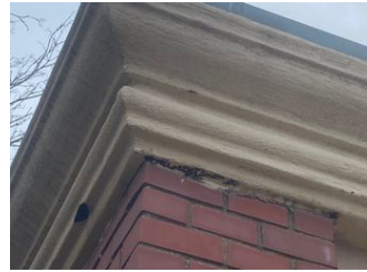
Stucco Eifs - Cornices decay
