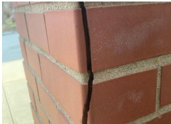
Brick Facade cracks
