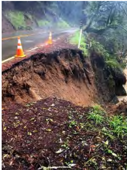
Figure 3.55: February 2017 Landslide on Lucas Valley Road
