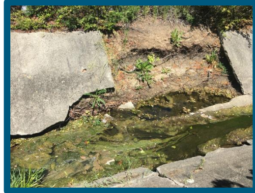
Concrete panels in need of repair
