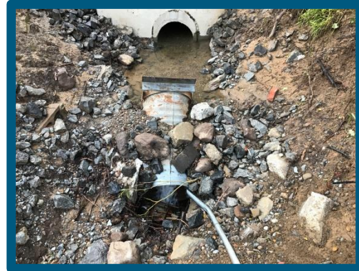
Drainage pipe blocked by debris
