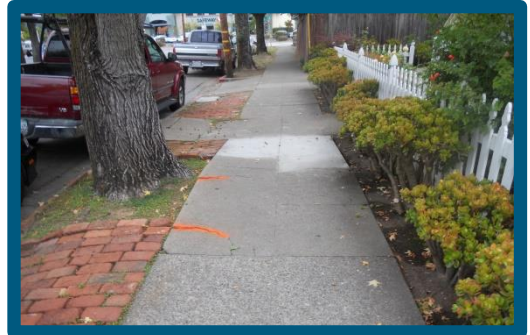
Displaced sidewalks in San Rafael
