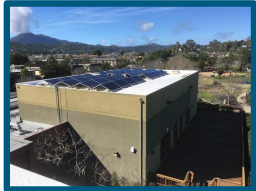
Solar panels recently installed on the Al Boro Community Center roof
