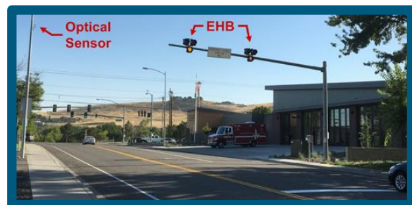
Example of an Emtrac System installed at an intersection
