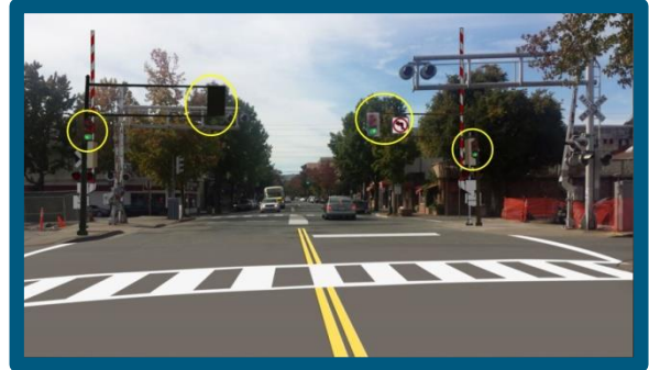
Queue Cutters recently installed at a SMART rail crossing on 4 th Street
