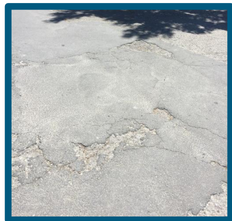
Pavement in the B Street Parking lot
