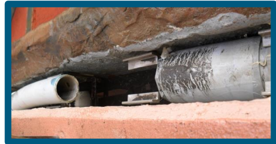
Pipe system and concrete at Court Street Fountain
