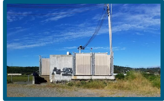
San Quentin pump station
