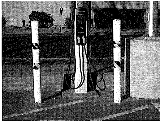
New Electric Vehicle Charging Station
