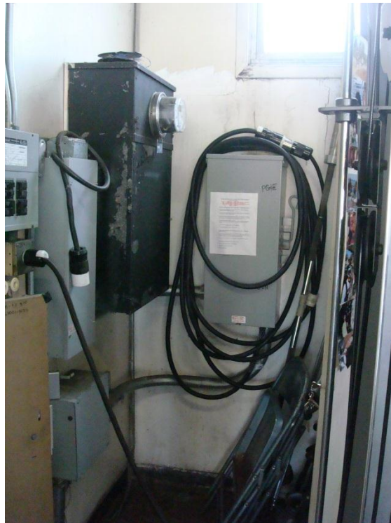
Figure E2: Manual Transfer Switch next to Main Meter Pedestal
