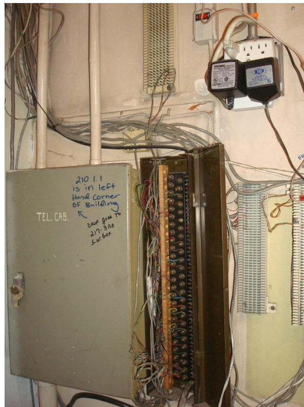
Figure E4: Telephone Equipment in Closet
