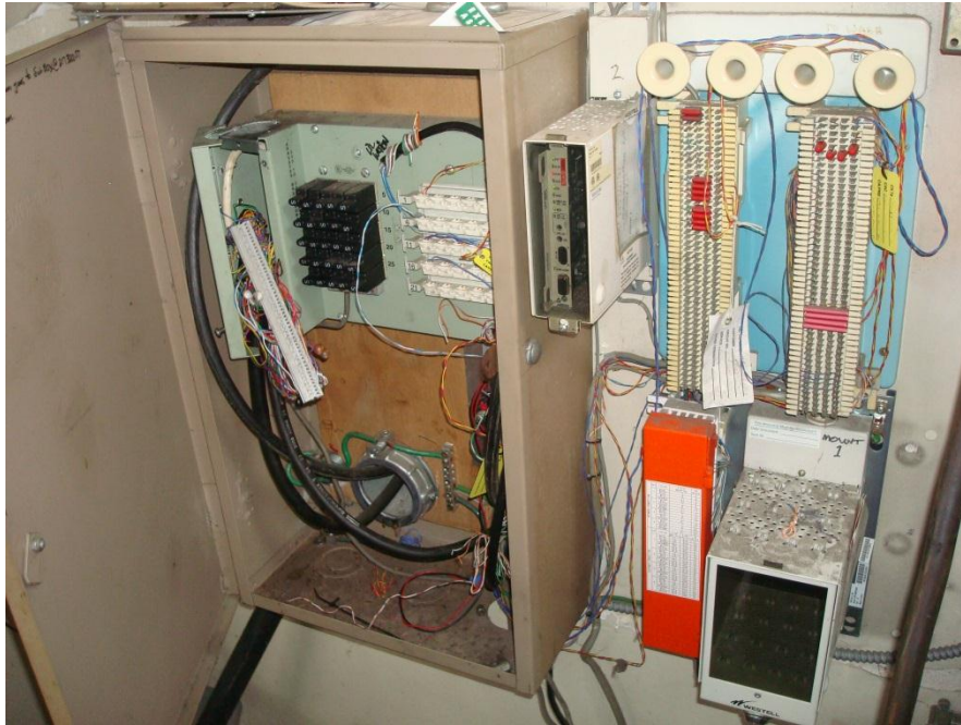
Figure E3: Low Voltage Equipment and Telephone Backboard
