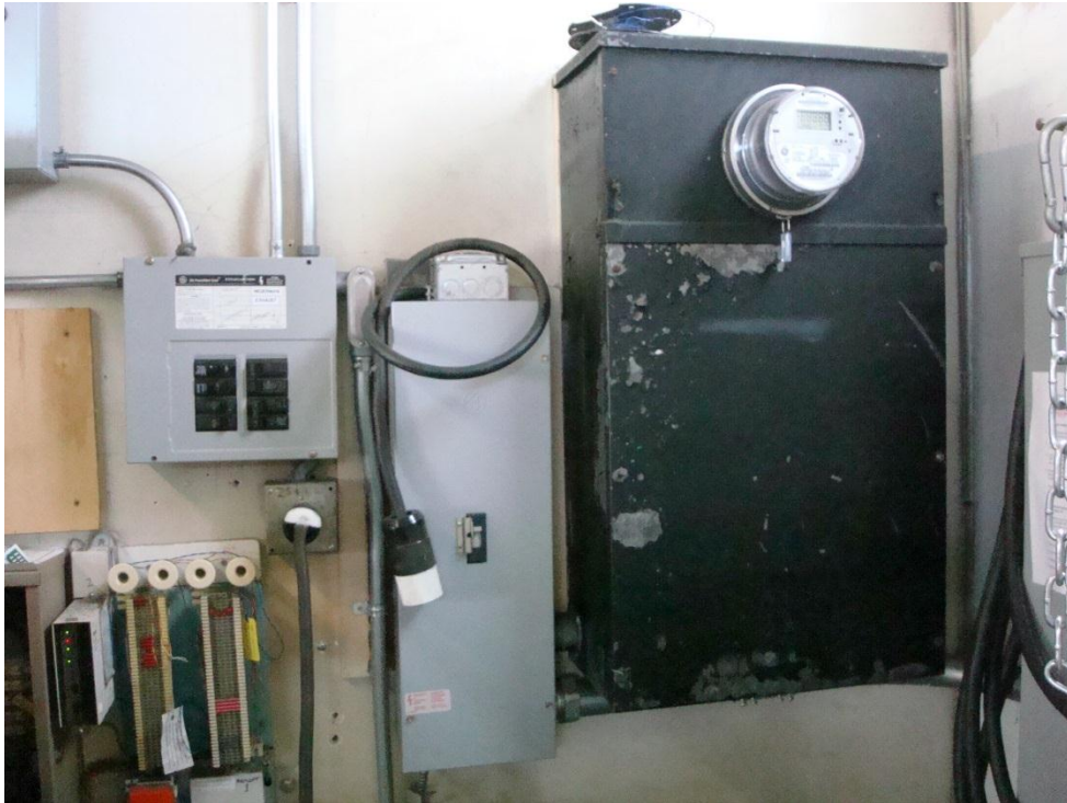
Figure E1: PG&E meter pedestal, main disconnect, and load center
