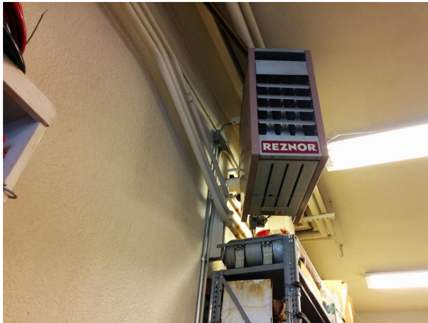
Figure M4: Force Air Unit Heater in Maintenance Bay
