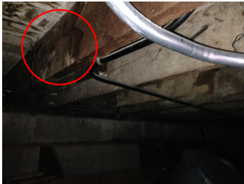
Photo 6: Station 51, Water Damage on Underside of Floor
