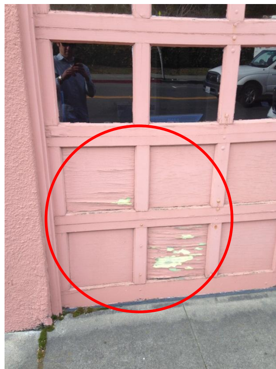
Photo 4: Station 51, Dry Rot Damage on App Bay Doors
