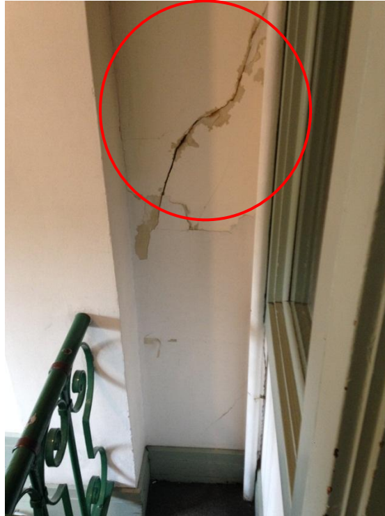
Photo 7: Station 51, Seismic Cracking in Plaster
