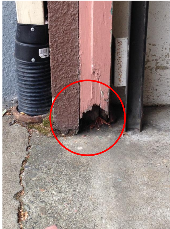
Photo 5: Station 51, Dry Rot Damage on Wood Studs
