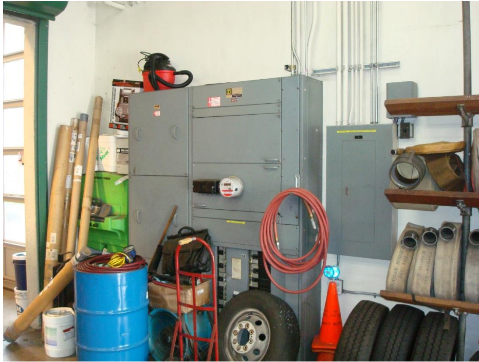
Figure E1: Main Switchboard and Panel "N" in Apparatus Bay
