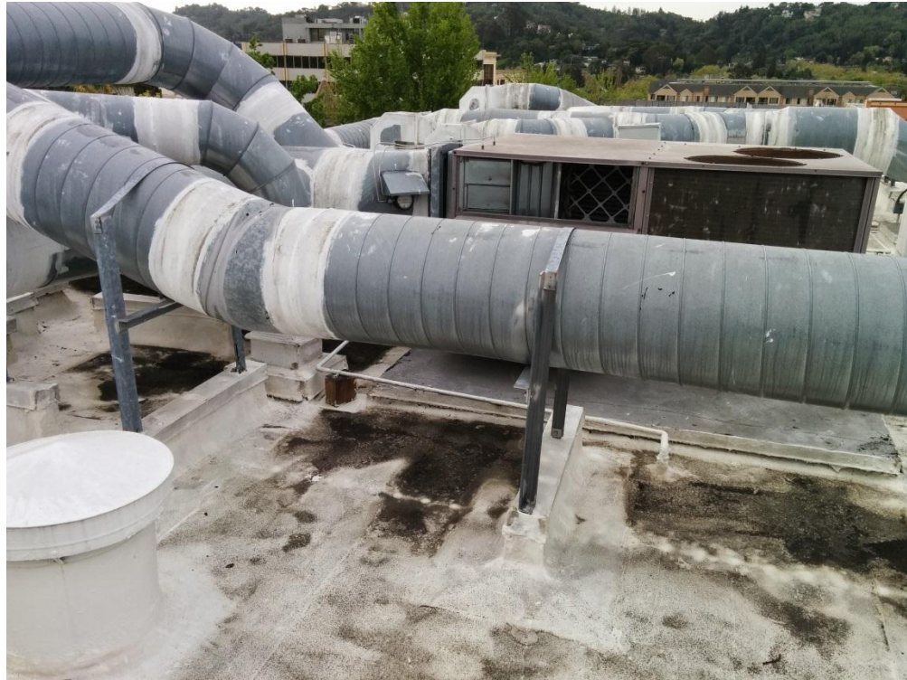
Figure M1: Main Building Rooftop Package Unit and Rooftop Ductwork
