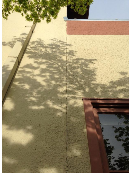
Photo 3: Station 51, Cracks in Perimeter Walls
