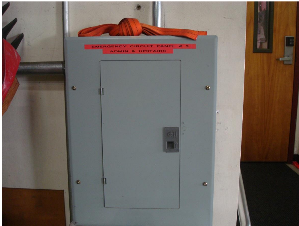
Figure E6: Emergency Panel in Apparatus Bay
