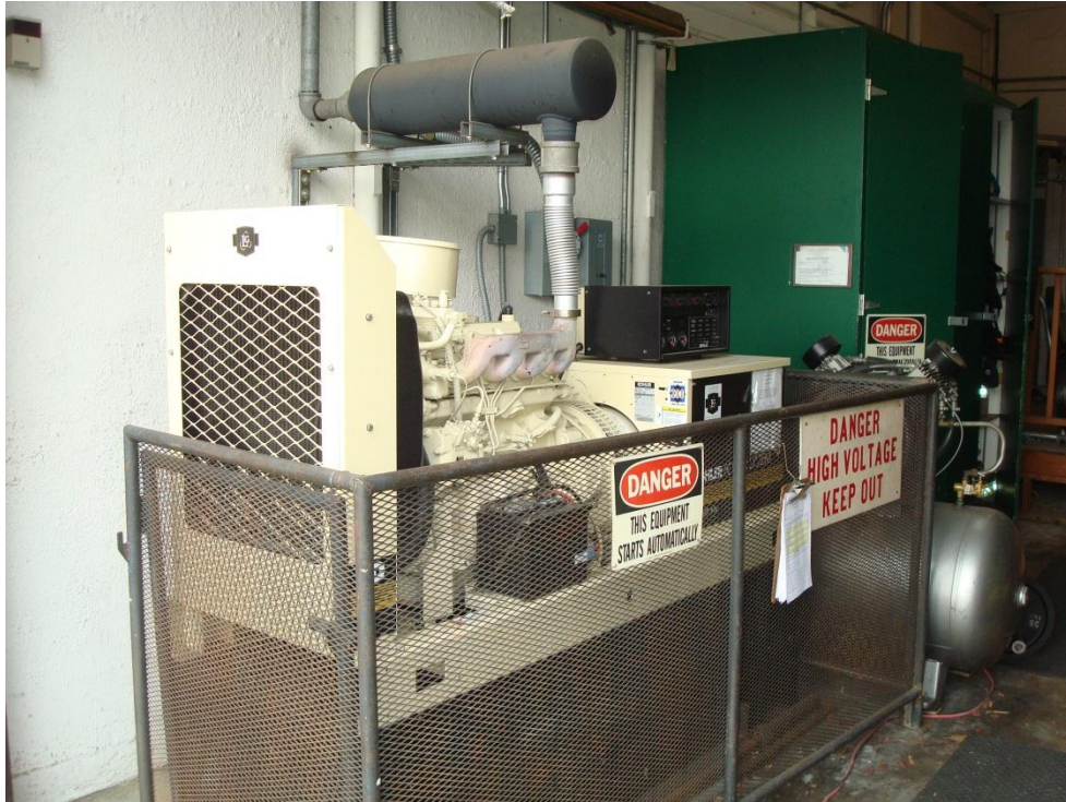
Figure E3: Emergency Generator System
