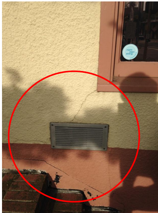
Photo 2: Station 51, Cracks in Perimeter Walls
