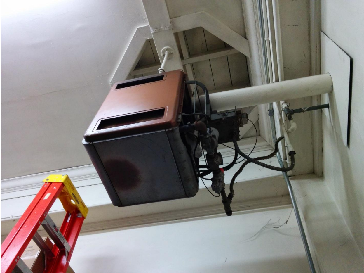
Figure M5: Force Air Unit Heater in Apparatus Bay
