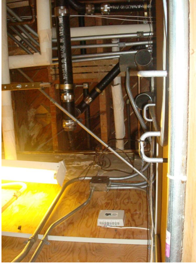
Figure E7: Leaking Sewage Piping In Telecom Room
