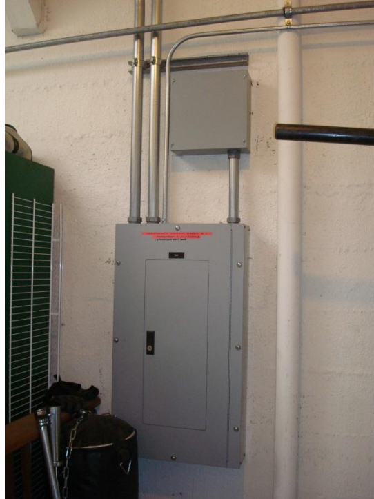
Figure E5: Emergency Panel “EM1” next to Generator
