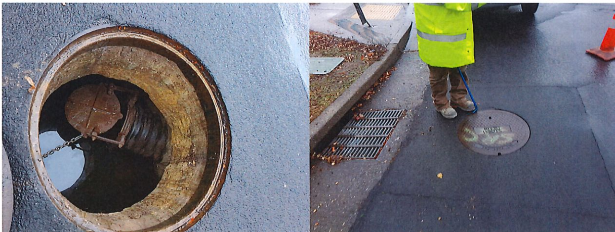
Figure 1: Los Gamos Road and Oleander Drive Manhole #14 (left) and adjacent inlet (right)
