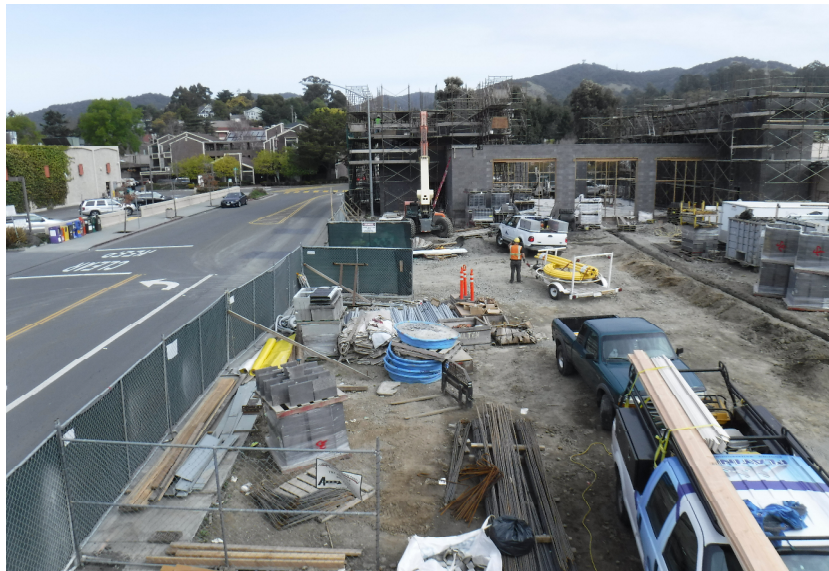
February progress picture – Looking North from Training Classroom to Fire Station Building
