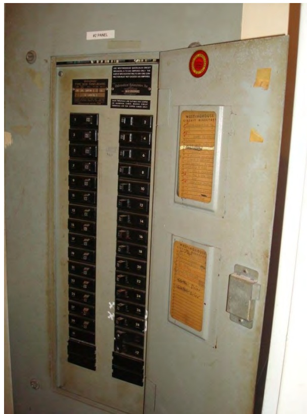
Figure E6: Branch Circuit Panelboard 'A' in Office Closet
