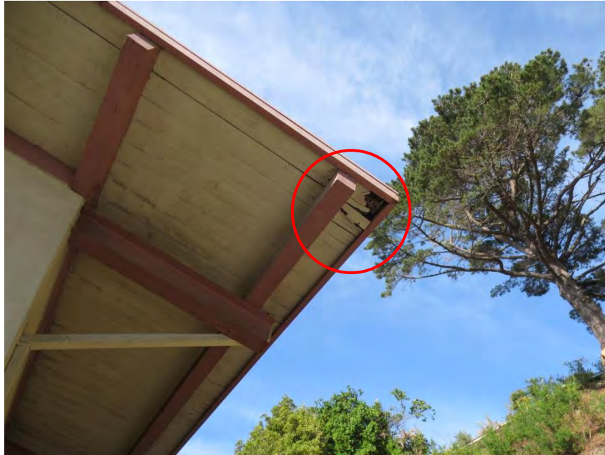
Photo 8: Station 55, Dry Rot in Roof Decking
