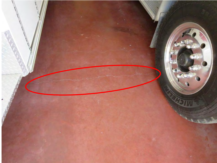
Photo 10: Station 55, Minor Slab Cracking in App Bay
