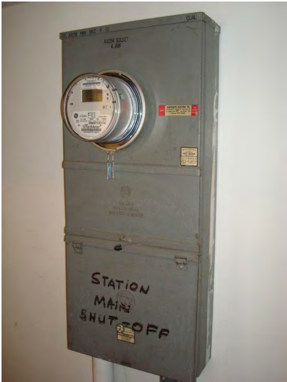
Figure E2: Main Service Meter and Pedestal
