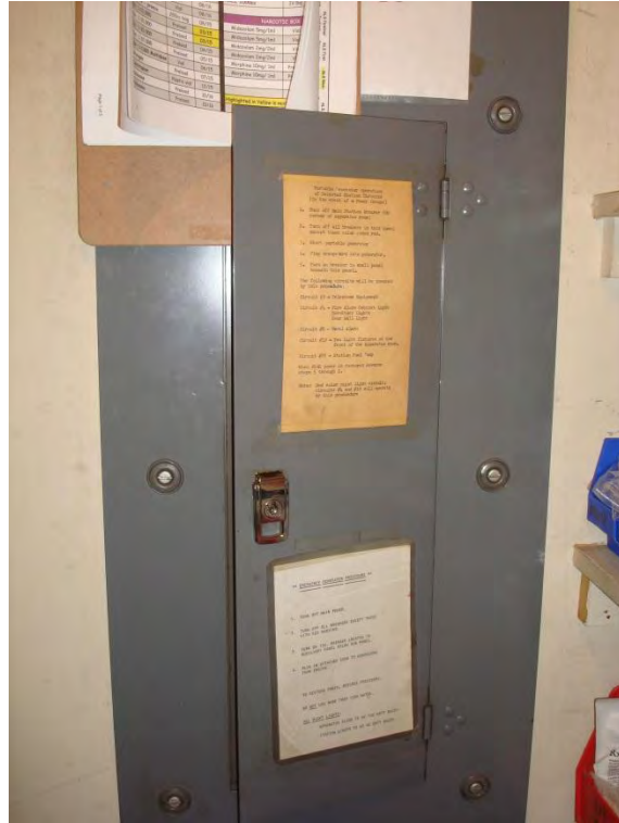
Figure E5: Branch Circuit Panelboard 'A' in Office Closet
