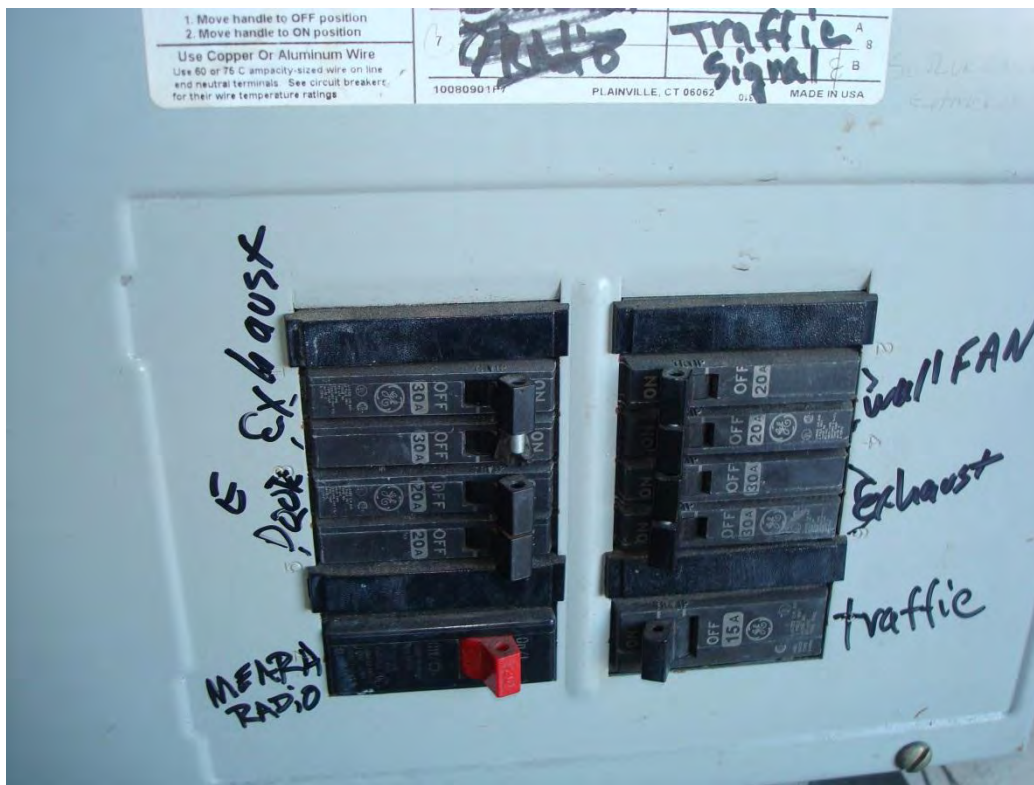
Figure E4: Load Center in Apparatus Bay
