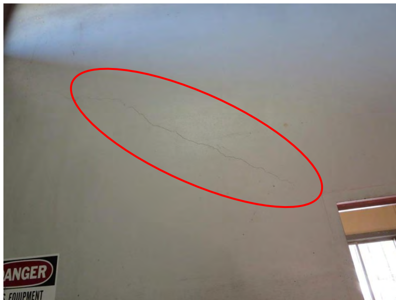
Photo 4: Station 54, Differential Settlement Cracking in App Bay
