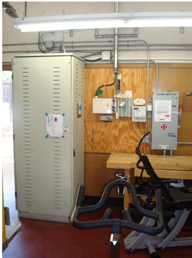
Figure E4: Communication Equipment Cabinet
