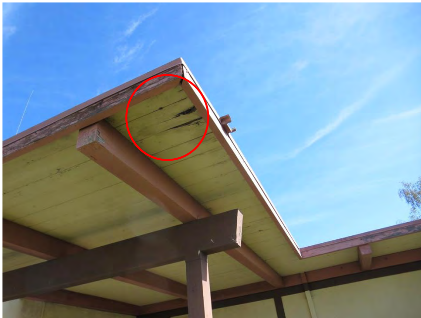
Photo 9: Station 55, Dry Rot in Roof Decking
