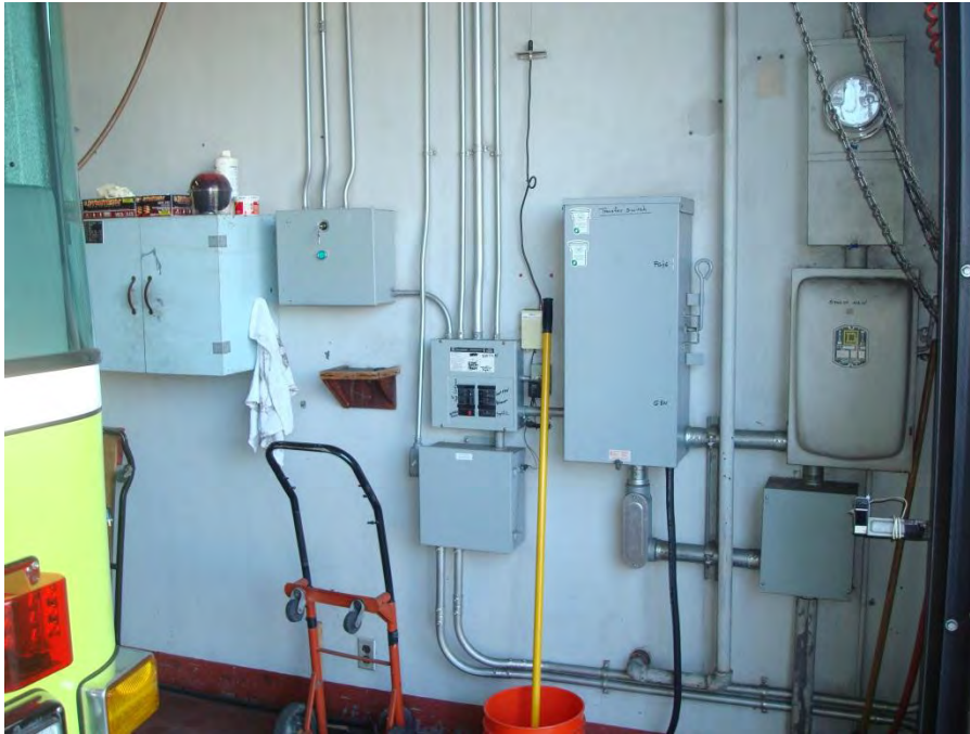
Figure E1: Incoming Electrical Service Equipment
