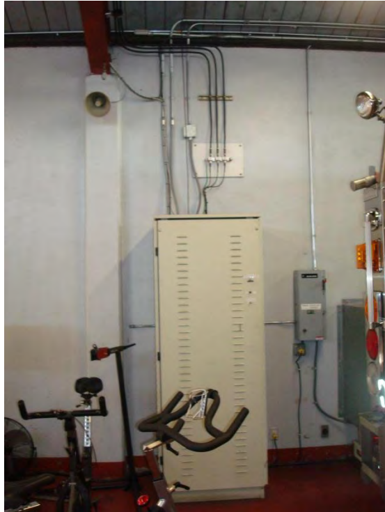
Figure E3: Typical Low Voltage Equipment Cabinet
