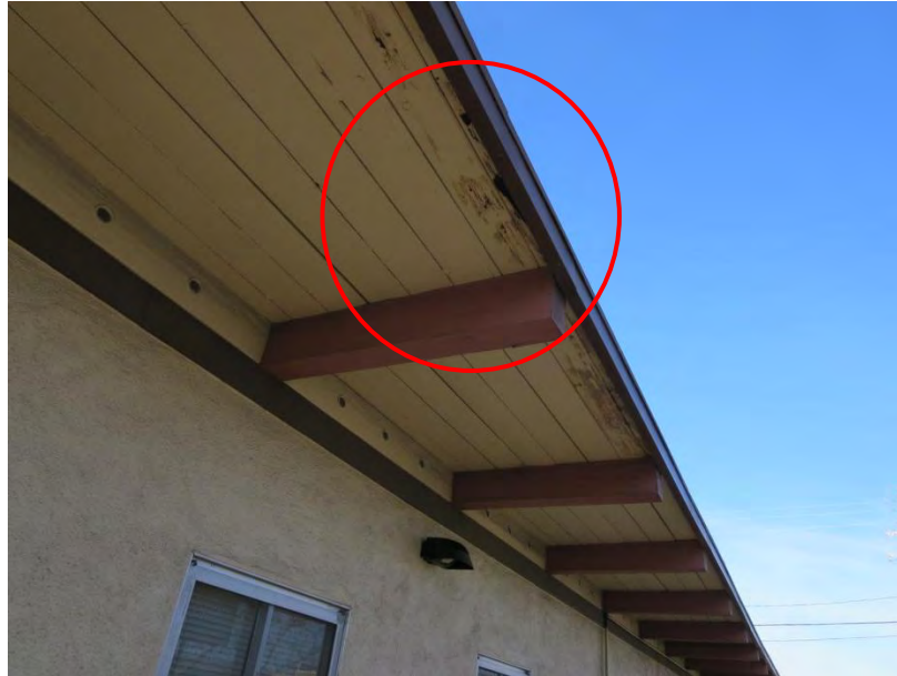
Photo 3: Station 54, Dry Rot in Roof Decking
