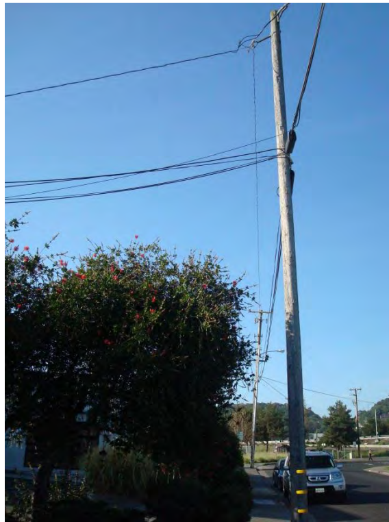
Figure E2: PG&E Utility Pole to Fire Station
