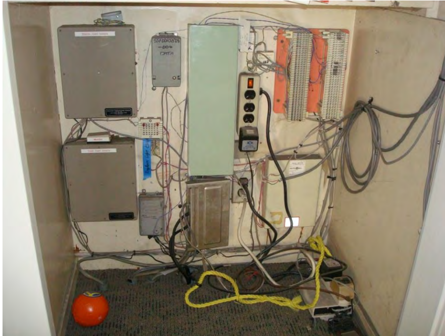
Figure E5: Telephone and Security Equipment in Office Closet
