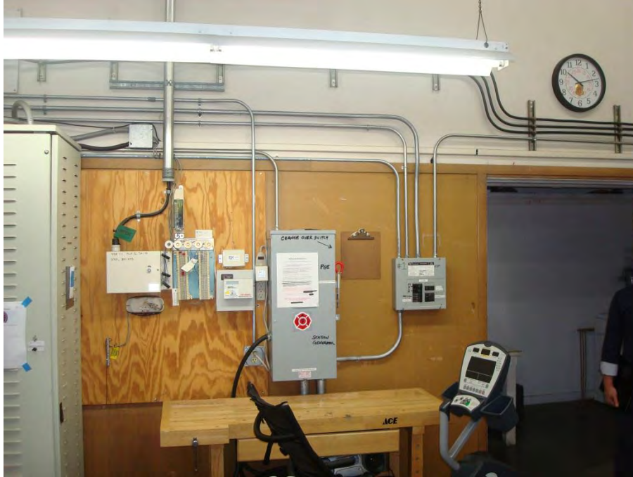
Figure E3: Manual Transfer Switch, Load Center, and Telephone Backboard
