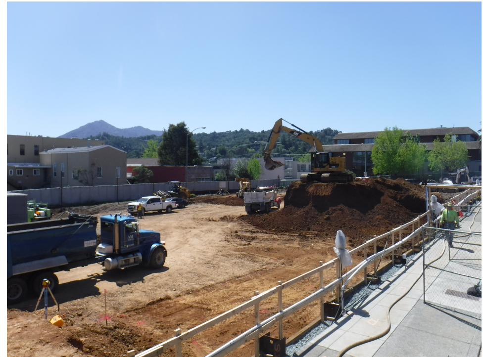
April progress picture – Overview of project site during haul off of the over excavated material
