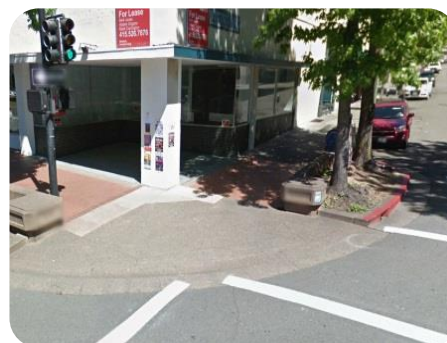
Fourth Street curb ramp needing ADA curb ramp installation
