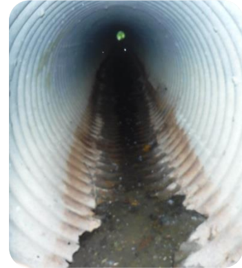
Pipe at Corrillo Drive to be replaced
