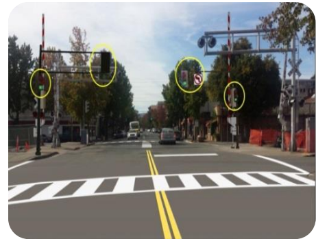
Queue Cutters recently installed at a SMART rail crossing on 4 th Street
