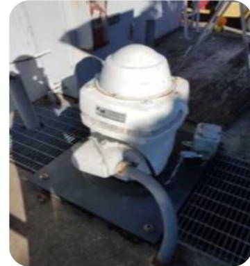
Cayes pump station control system to be updated
