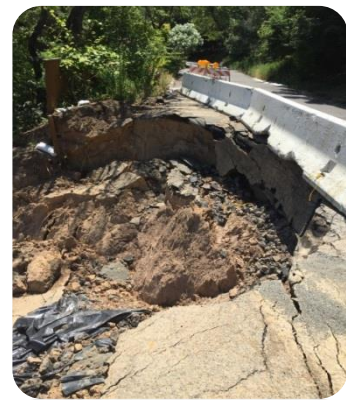
70 Irwin slide damages
