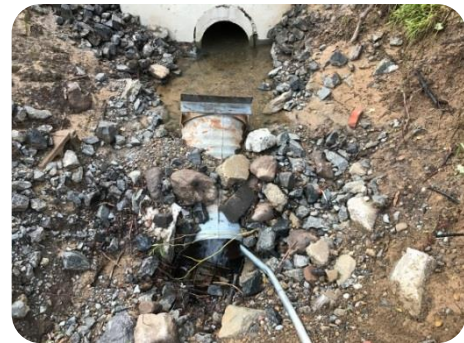
Drainage pipe blocked by debris
