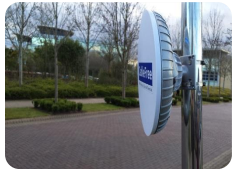
Example of microwave system
