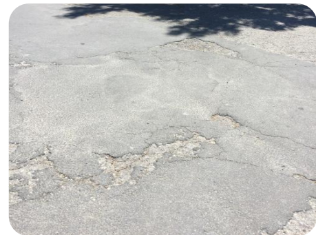
Pavement in the B Street Parking lot
