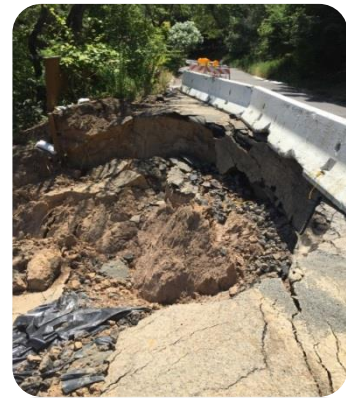
70 Irwin slide damages
