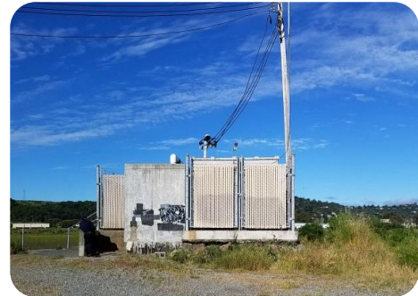
San Quentin pump station
