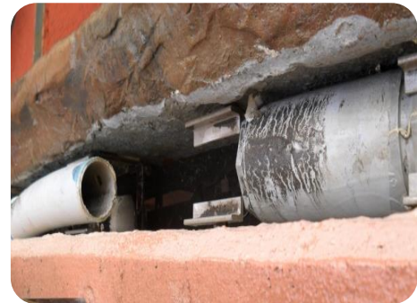
Pipe system and concrete at Court Street Fountain
