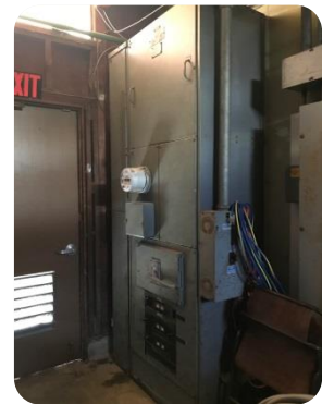
Terra Linda Pool House electrical panel systems
