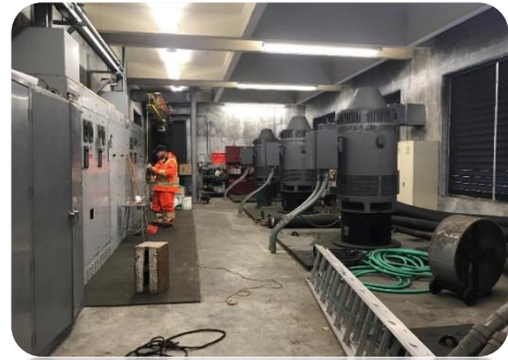
North Francisco Pump Station
