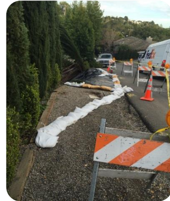
80 Upper Toyon slide damage
