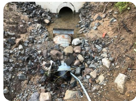
Drainage pipe blocked by debris
