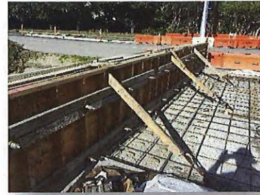
West side bridge deck barrier wall on the City of San Rafael, Freitas & Las Gallinas Intersection project— Inspection performed by Coastland
