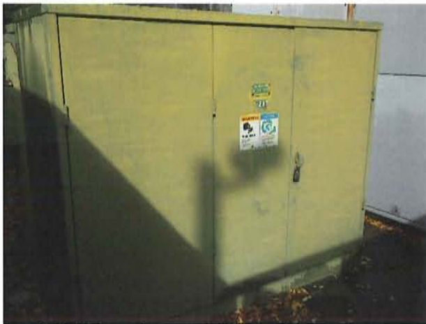
9. PG&E Transformer T-297 within Enclosure
