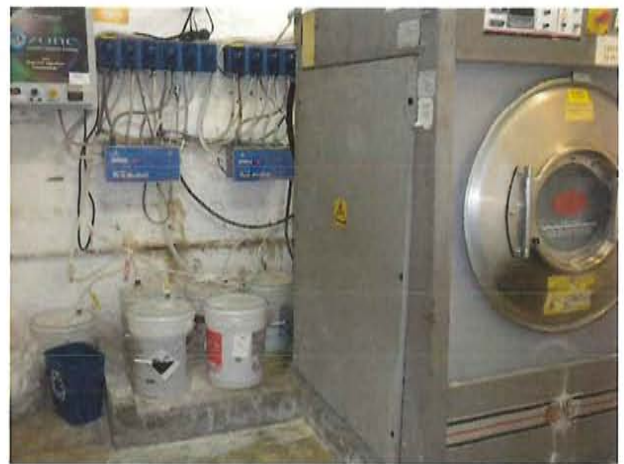
24. Laundry Chemicals on Corroded Concrete Slab in Housekeeping Area
