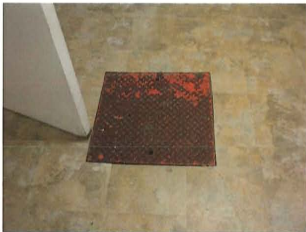
23. Covered Floor Drain in Housekeeping Area within North Tower Sub-Basement
