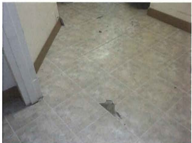
22. Damaged Flooring in Housekeeping Area within North Tower Sub-Basement
