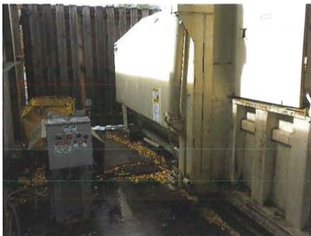
11. Trash Compactor Unit within Enclosure, Water on Pavement Due to Rain
