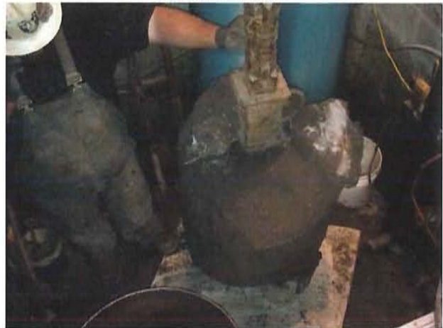
28. Hydraulic oil impacted soil encountered during jack hole enlargement
