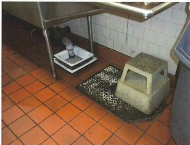
21. Grease Trap in Restaurant Kitchen Floor
