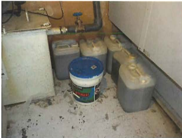
25. Oil-Water Separator Units and Stored Oil within North Tower Elevator Room
