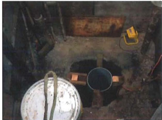
34. Top view of PVC secondary casing in elevator pit
