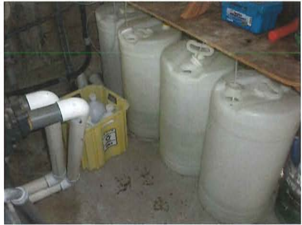
14. Pool/Spa Chemicals Stored within Enclosure
