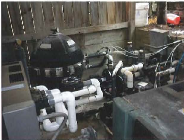
15. Pool Equipment within Enclosure
