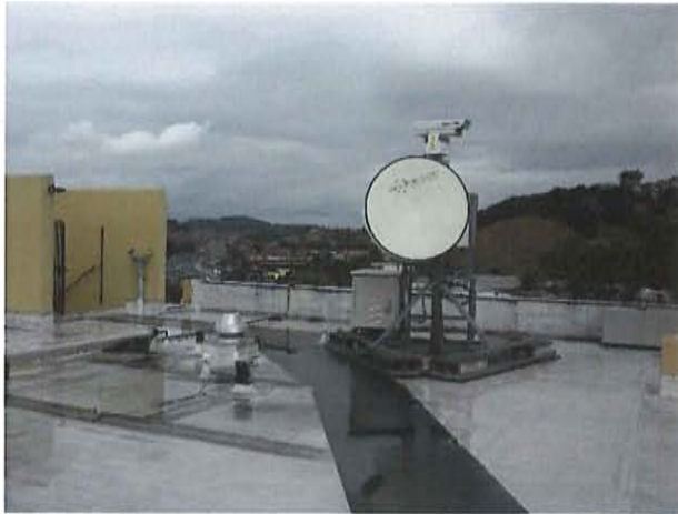
19. Antenna Equipment on North Tower Roof
