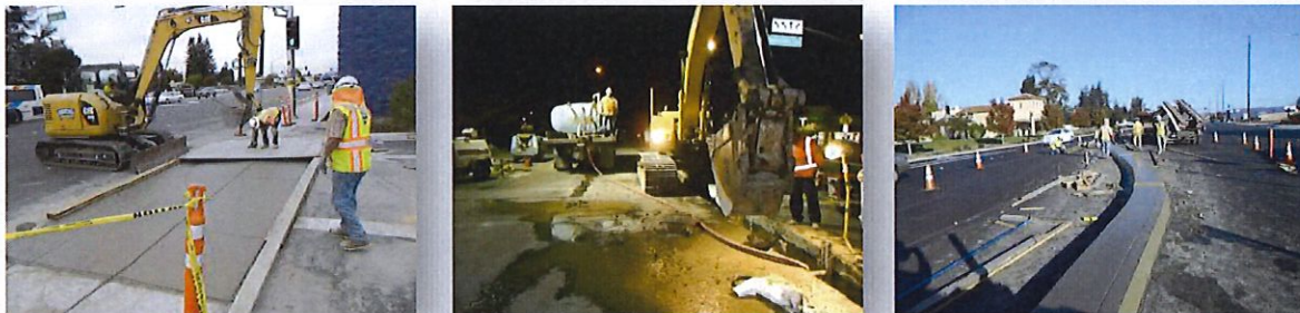
City of Santa Rosa: Santa Rosa Avenue Road Widening Project—Construction Management & Inspection performed by Coastland
