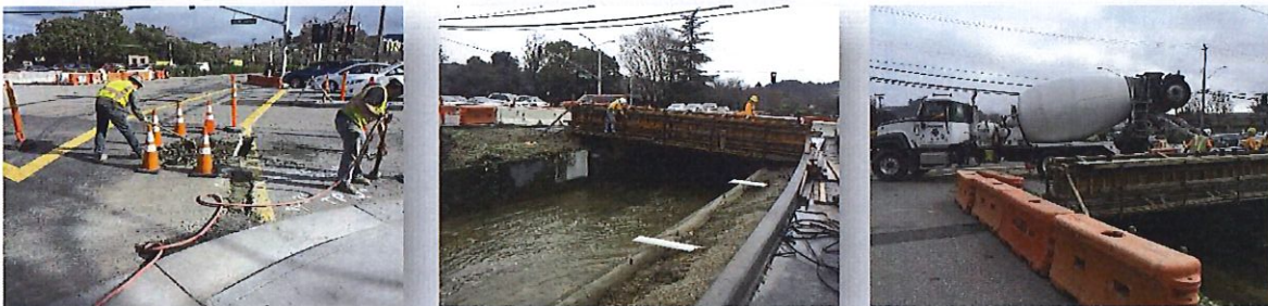
City of San Rafael: Freitas & Las Gallinas Intersection Improvements Project—Construction Inspection performed by DeWayne White
