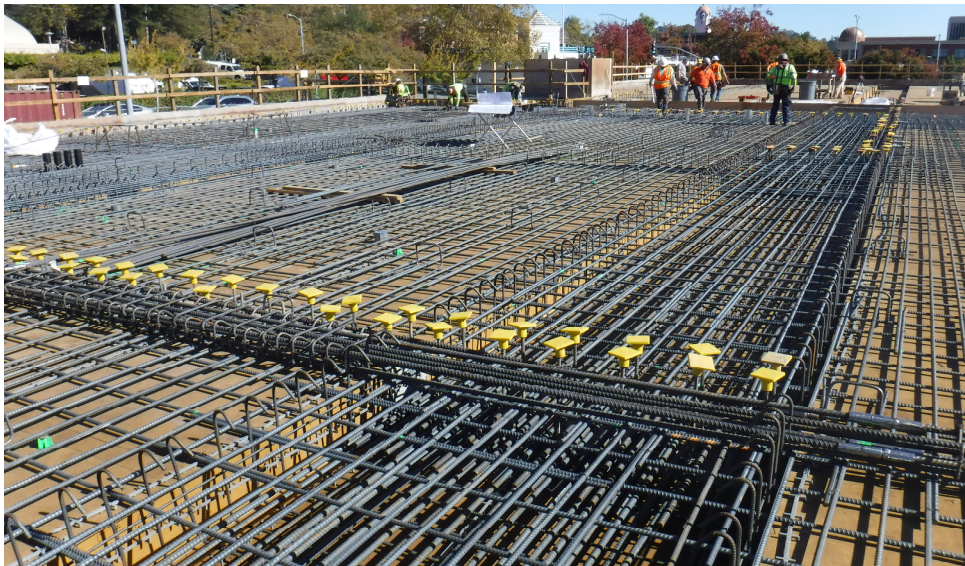
October progress picture – layout of first floor rebar and beams in preparation for concrete.
