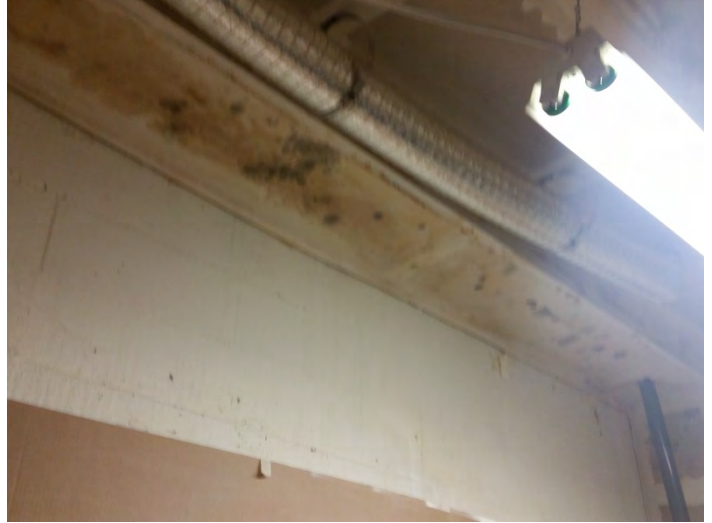
14. Mold on ceiling drywall inside of the paint room
