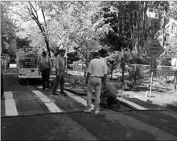
A Public Works crew installs a speed hump to slow neighborhood traffic.
