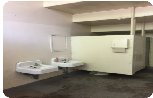
Current conditions of Albert Park Ball Field restrooms
