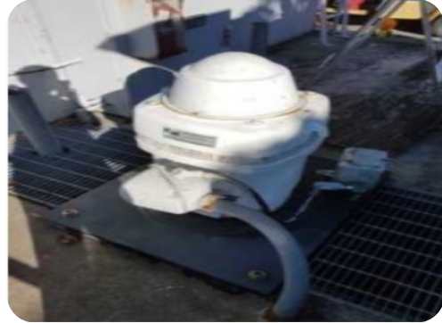
Cayes Pump Station Control System to be updated
