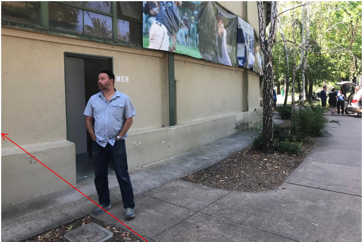
Approximate location of door for one ADA compliant, family-style restroom. Similar restroom on opposite side of the bleachers as well.
