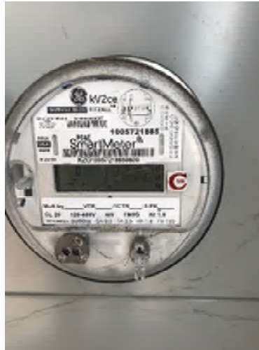
Main Electrical Service Meter
