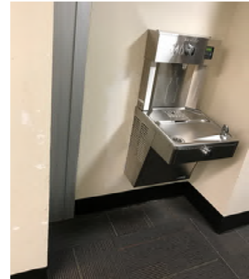
3.4 Level 1 Drinking Fountain
