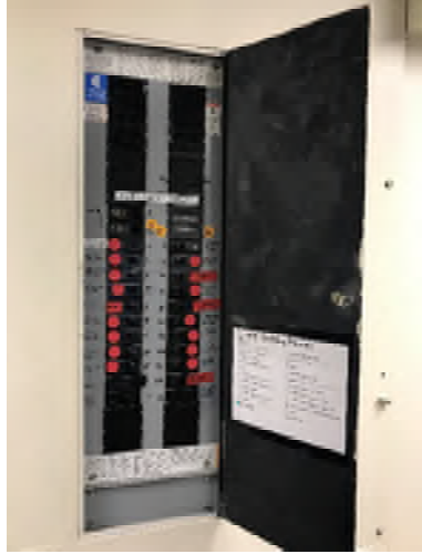
Original Branch Panels
