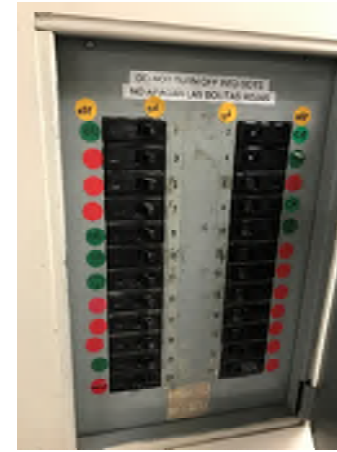
Circuit Breaker Controls
