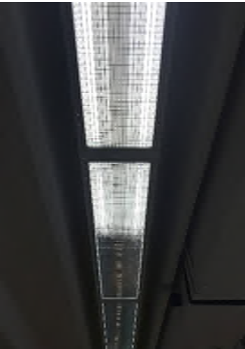
Stack Area Open Lighting
