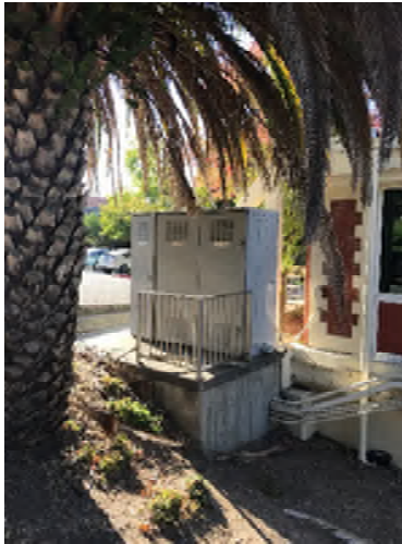
Main Electrical Service Panel
