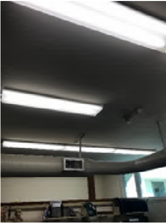
Interior Lensed Lighting
