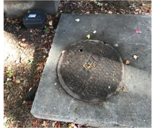
1.3 Perimeter Drain Sump Pump Location
