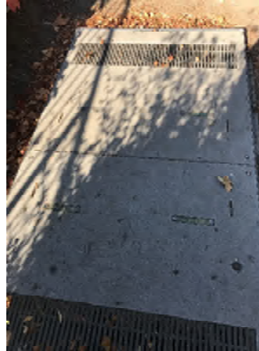
Utility Transformer Vault
