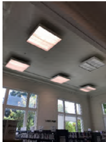
Original Bldg. Lighting
