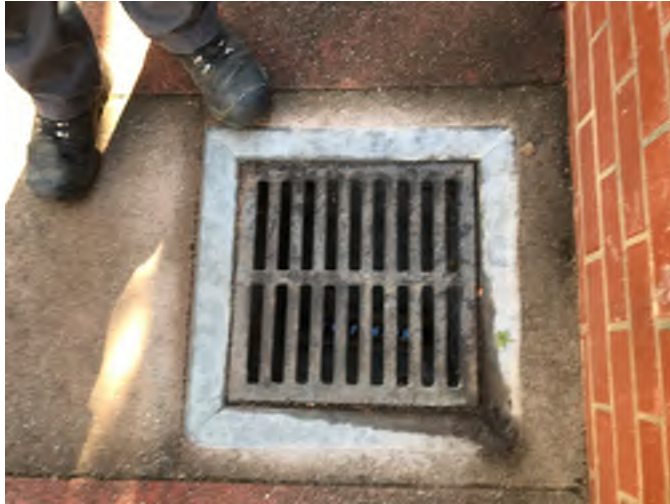
1.1 Sewer Main cleanout
