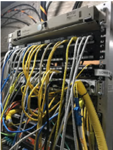
Older Cat 5 Cabling
