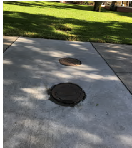
1.2 Sewer cleanouts at Fifth Ave Sidewalk. Entrance to the library can be seen on the background.
