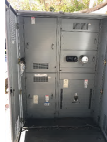
Main Meter / Main Section 1
