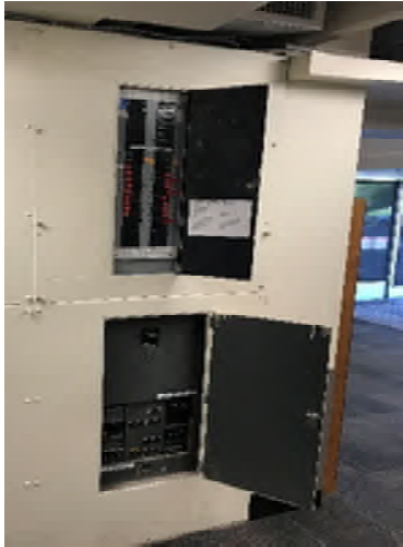
Original Distribution Panel (At front entry Lobby)
