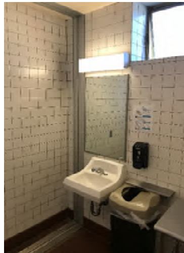
Surface Mounted Lighting
