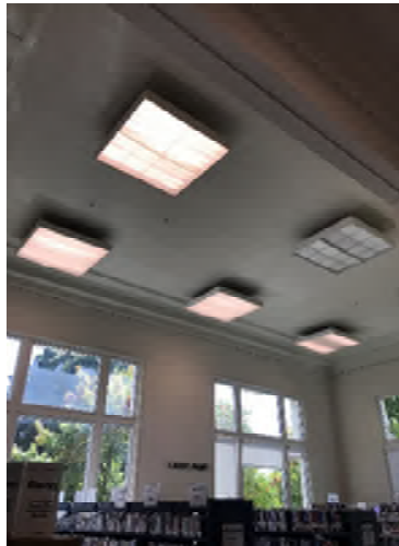
Original Bldg. Lighting
