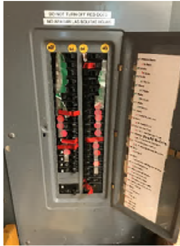
Original Branch Panels
